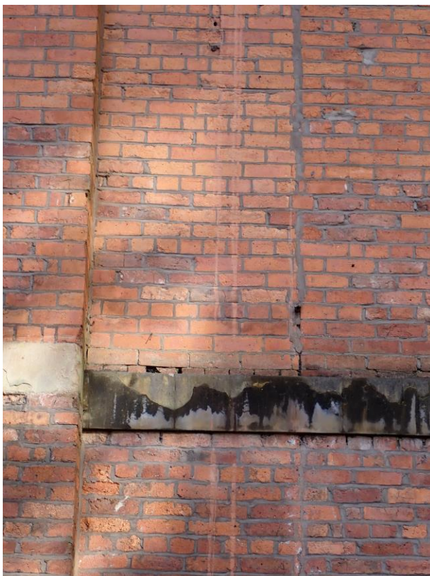
Photograph 2. Cavities within the brickwork on the southern aspect of the building.
