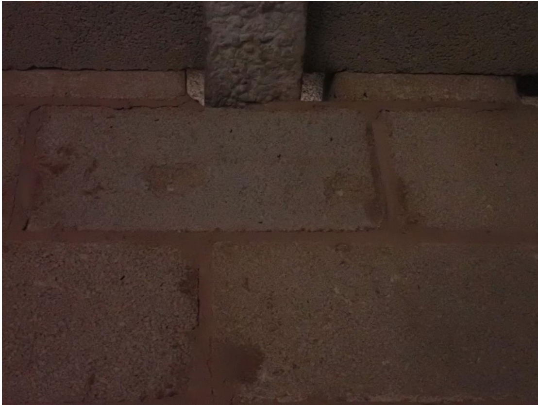
Photograph 9. Bat droppings identified on a breezeblock wall.
