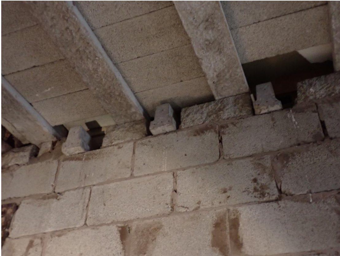
Photograph 5. The breezeblock ceiling, showing gaps above the wall plate.
