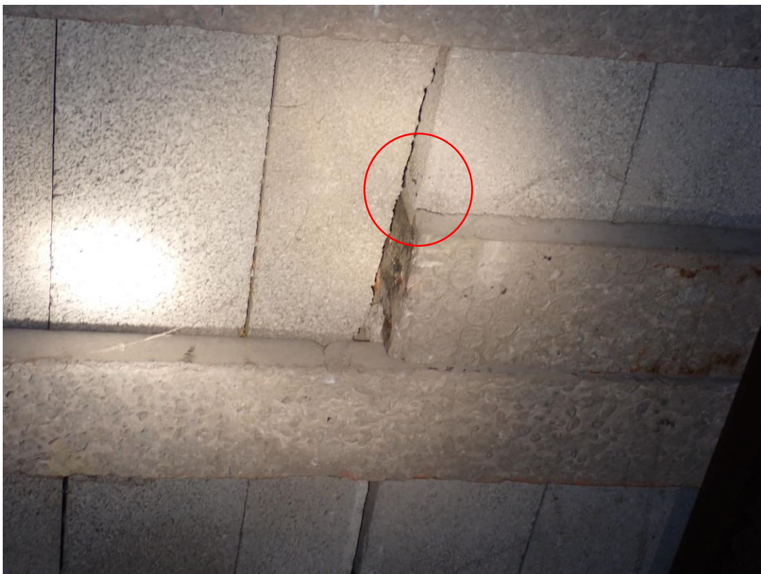
Photograph 10. Bat droppings leading into a crevice in the ceiling.
