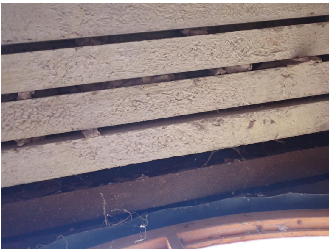
Photograph 12. Crevices in the brickwork above the windows.
