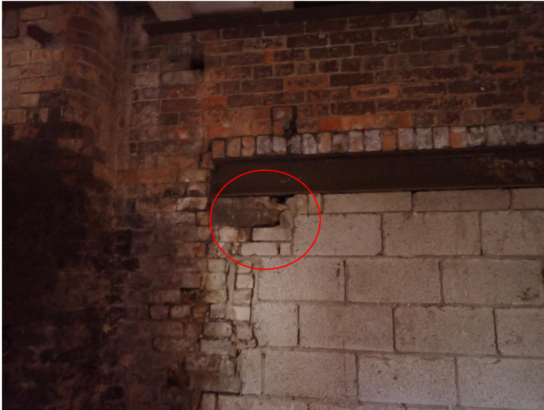
Photograph 7. Cavities within the brickwork.
