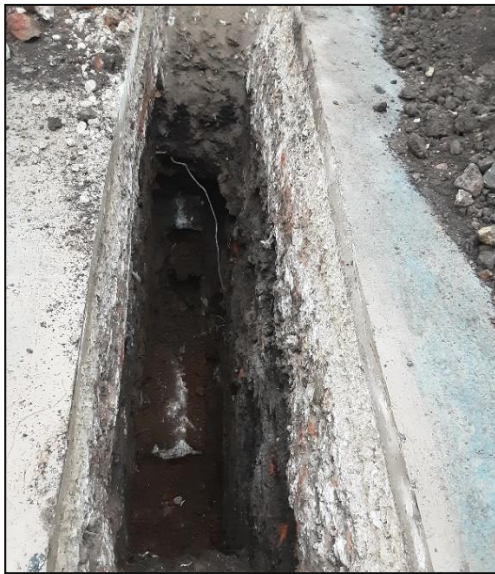
Figure 4-1 Hardstanding underlain by light grey gravel within top 0.5m followed by dark brown sandy gravel. Note concrete obstruction extending across the base of the pit at 3.5mbgl (TP22/02).
