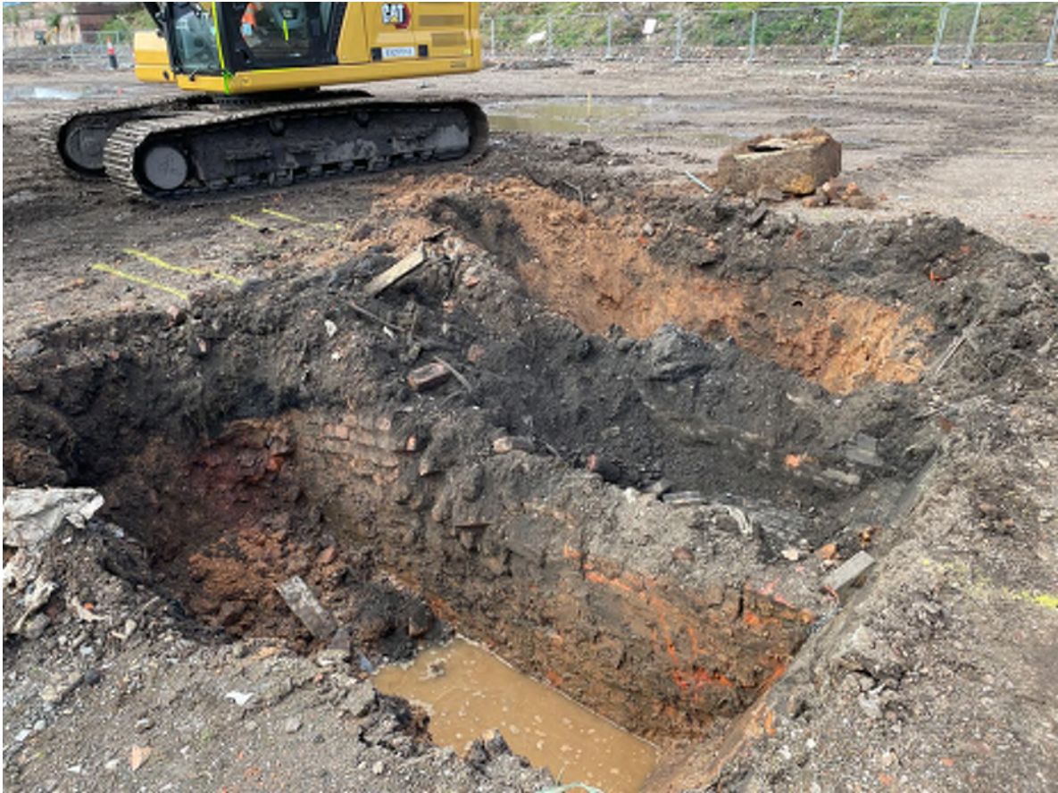
Photograph 2: – CS3 exposing carriage shed foundations with perched water inside the structure
