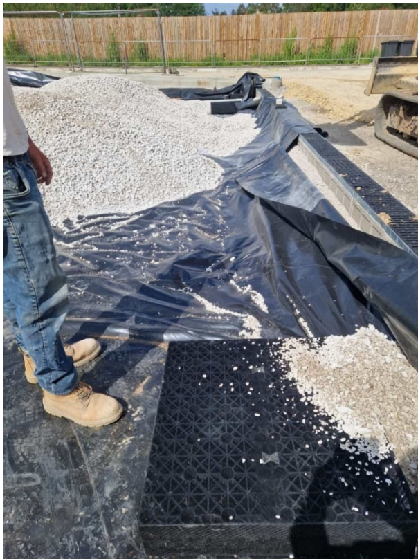
Photo 3 – Macro construction. Distribution box
