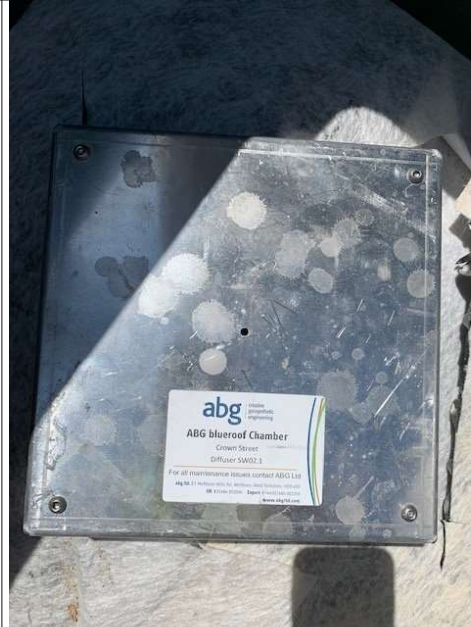
Close up image of diffuser (at C4 outfall) – as shown in drawing Z2- NRA-G240- De- Gd-009
