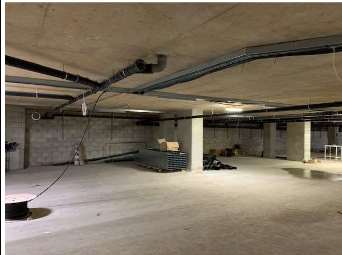
Photo 19 – B1 Level Underslung Drainage From Blue Roof Attenuation Crate To Main Drainage Spine
