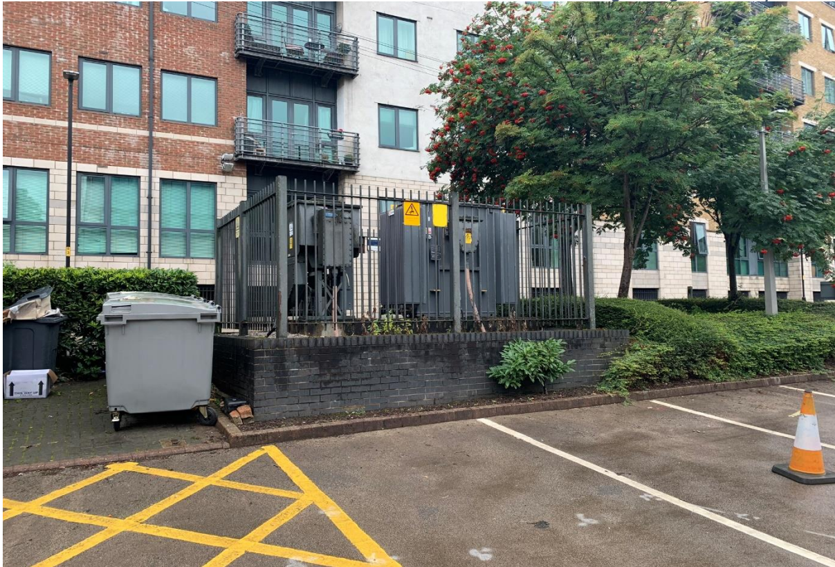
Plate 7 – Electricity Substation in West and Centre of Site
