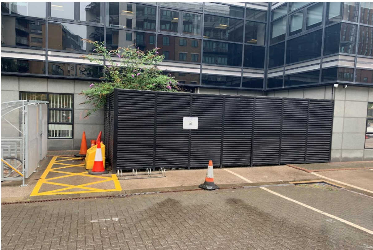
Plate 4 – Mechanical Plant in East of Site
