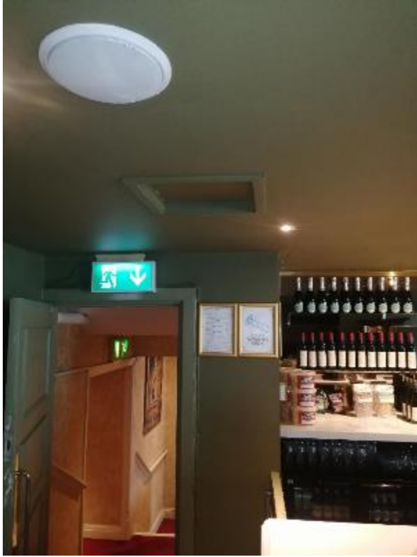
Existing Location Cloud AP25
