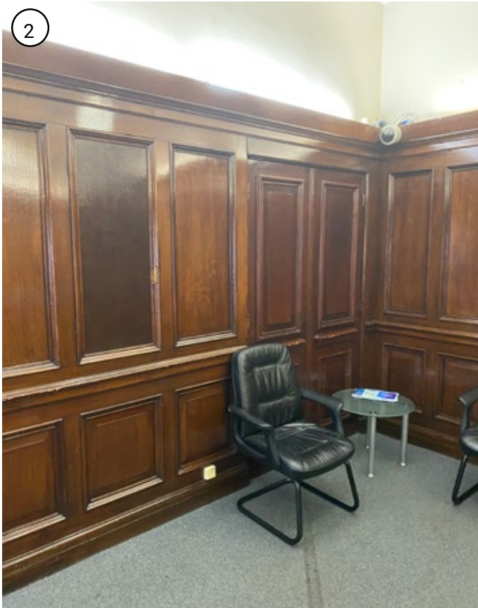
Original Paneling - Localised breakthroughs
