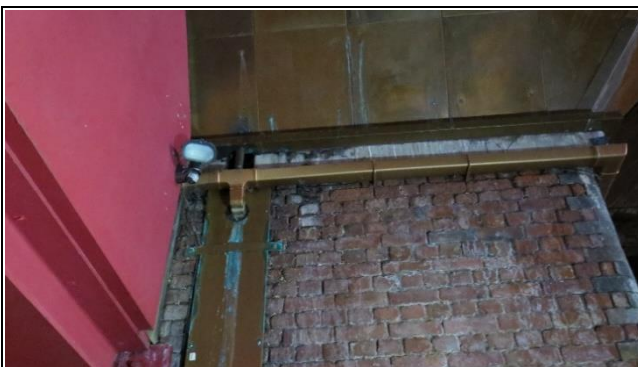
East Wall of Arch 4 with Discoloured Copper Panelling, Double Gutters and Downpipe
