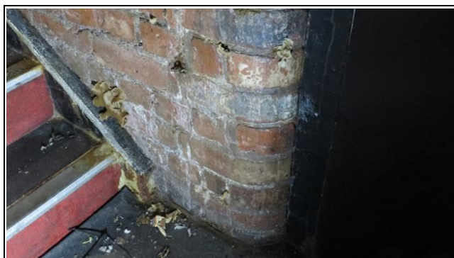
Dry Rot on Rear Staircase
