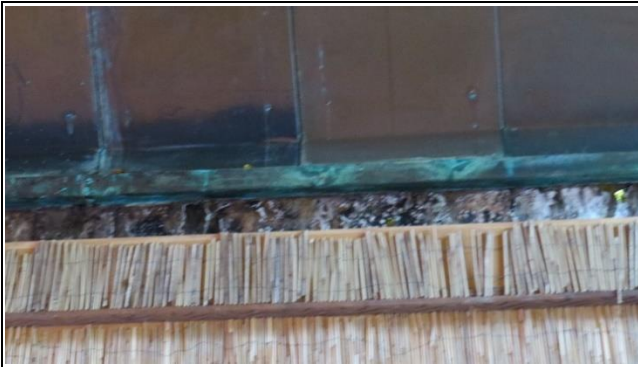
Evidence of Overflowing Gutters
