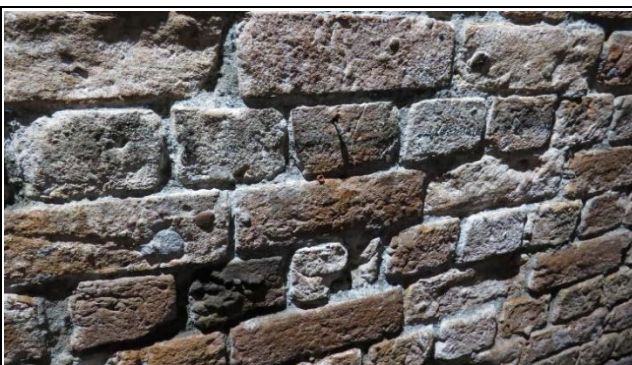
Spalling Brickwork in Basement
