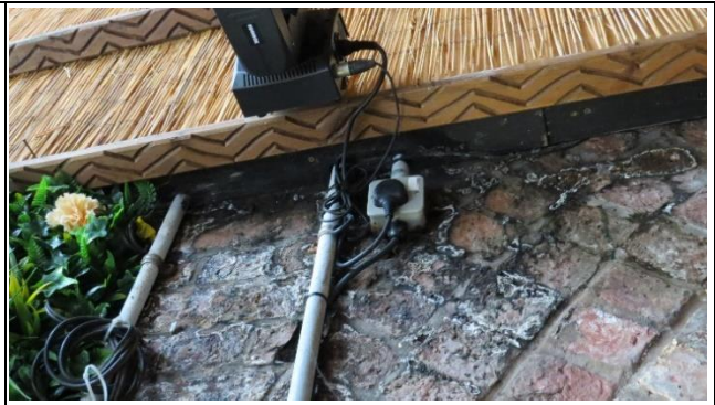
Impact of Water Ingress on Brickwork
