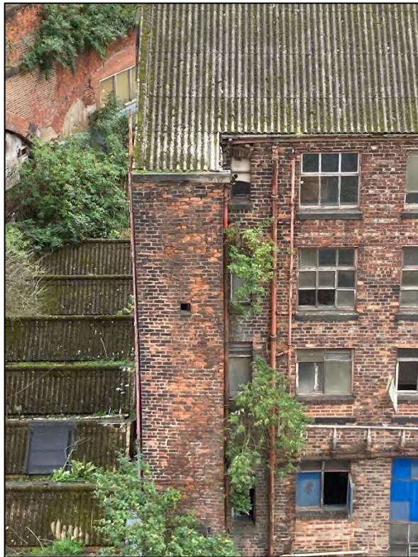
Figure 2: Example of cavity in brick work of building. Open windows can also be clearly seen.
