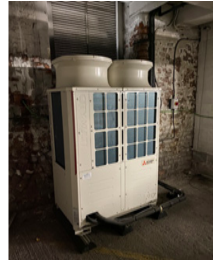
3.3.3 Existing condensing unit
