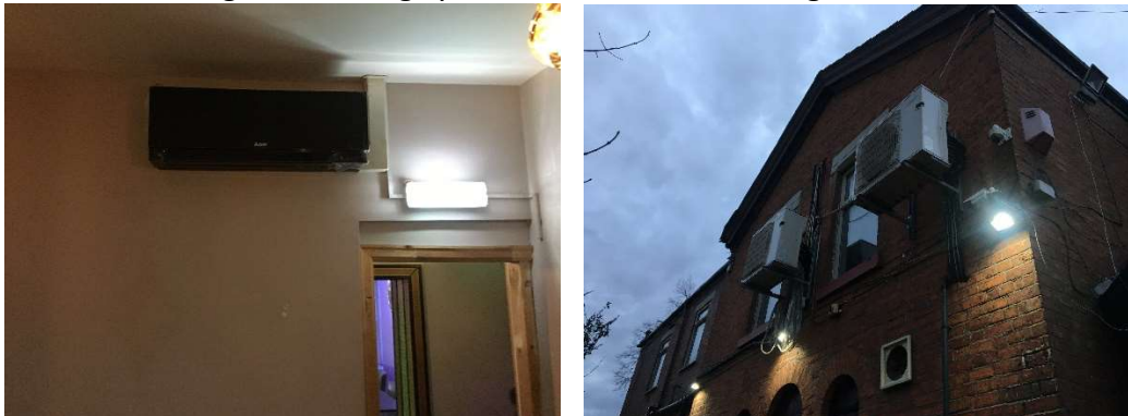
External units of air-conditioning/heating system
