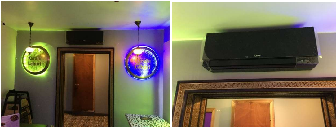
Air conditioning and heating system internal units throughout the restaurant
