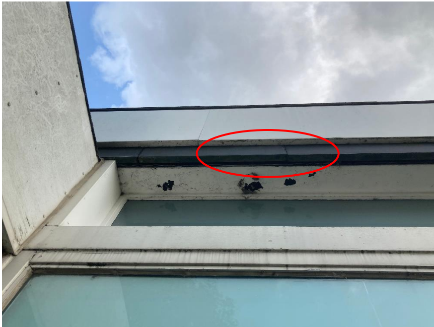
Photograph 2 - Potential bat roosting crevice at the front of the building
