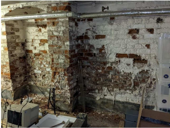
Figure 2-13 Station Bldg basement – masonry degradation due to moisture ingress
