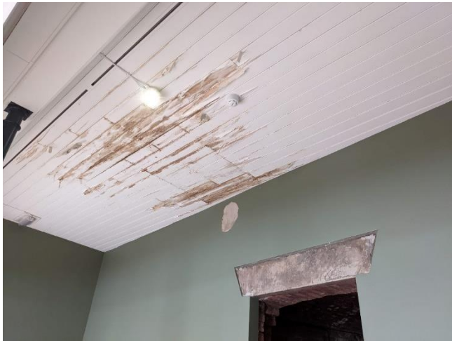
Figure 2-11 Water damage to ceilings in Station Building
