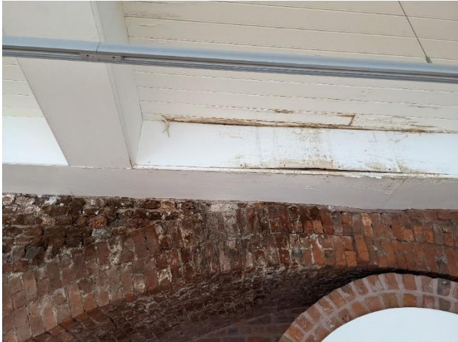
Figure 2-6 Flattening of crown of arch 4A
