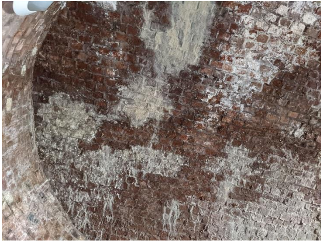
Figure 2-9 Staining due to extensive water ingress – arch 3A
