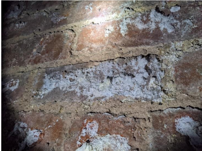
Figure 2-10 Efflorescence to face of masonry – arch 5B
