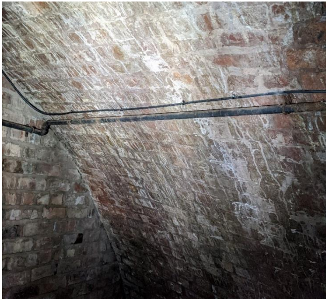
Figure 2-12 Staining due to water ingress – arch 5B
