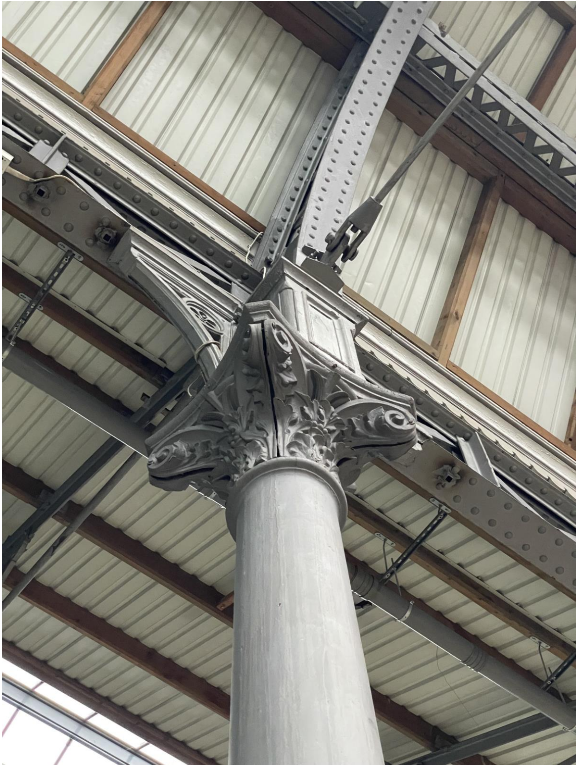
Figure 93: Detail of one of the original decorative Corinthian cast iron capitals.
