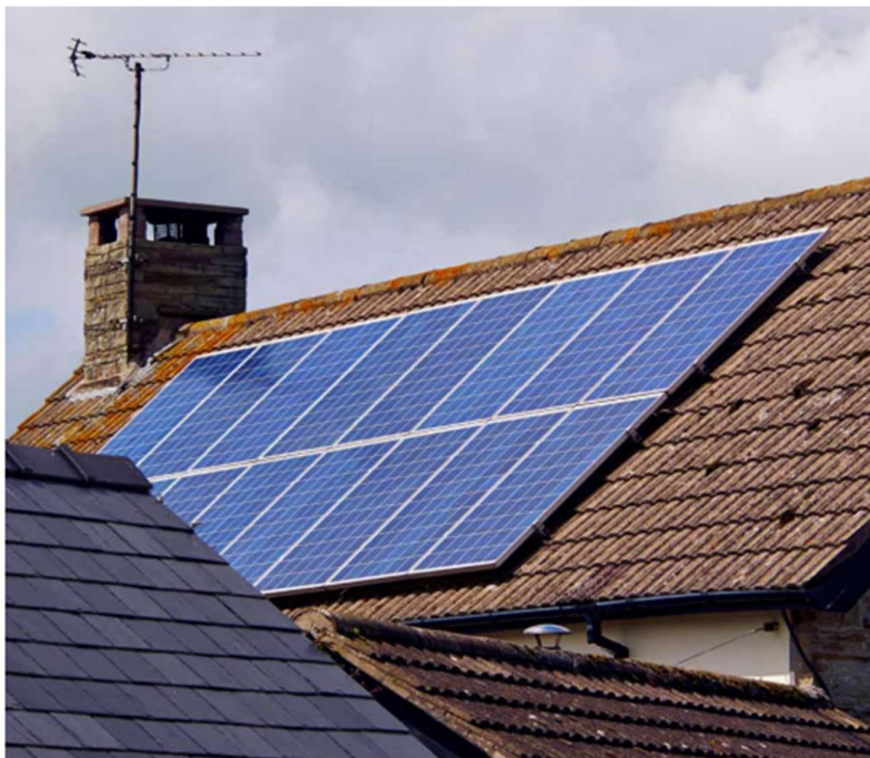
Photograph of example solar panels, coloured blue
