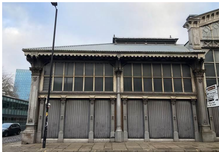
Figure 60: The western section of the south elevation, showing the original cast iron structure and glazed upper framework. The lower parts have had their cast iron railings removed and replaced with modern corrugated metal sheeting.
