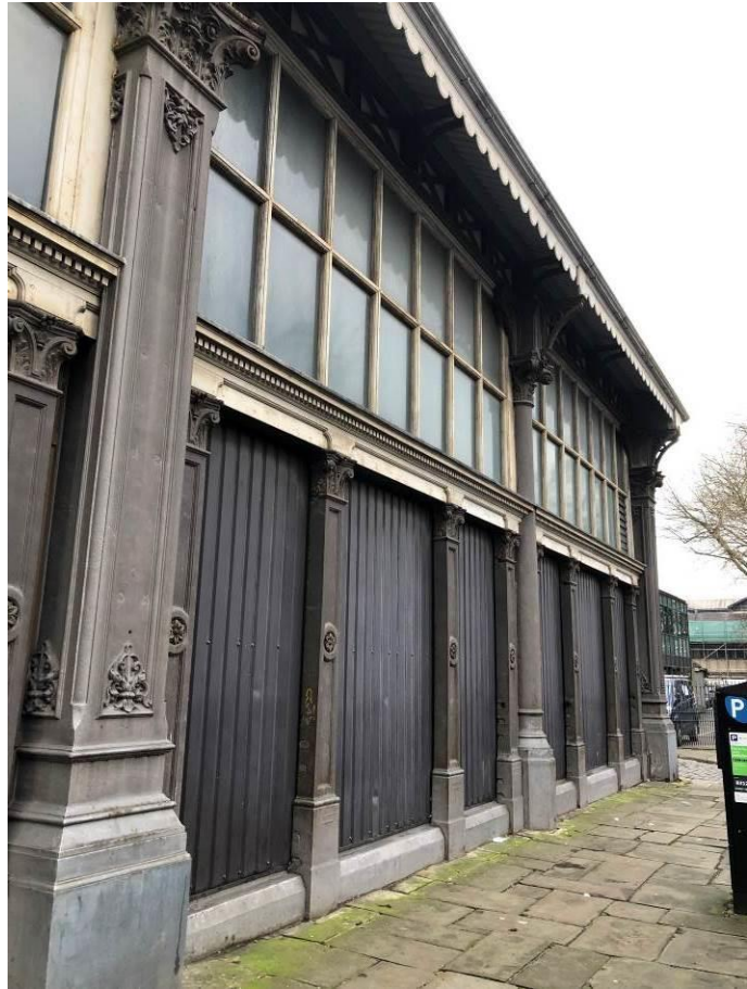
Figure 65: The western part of the north elevation, showing the modern corrugated sheeting replacing the original cast iron railings, with original timber and glazed framework above.
