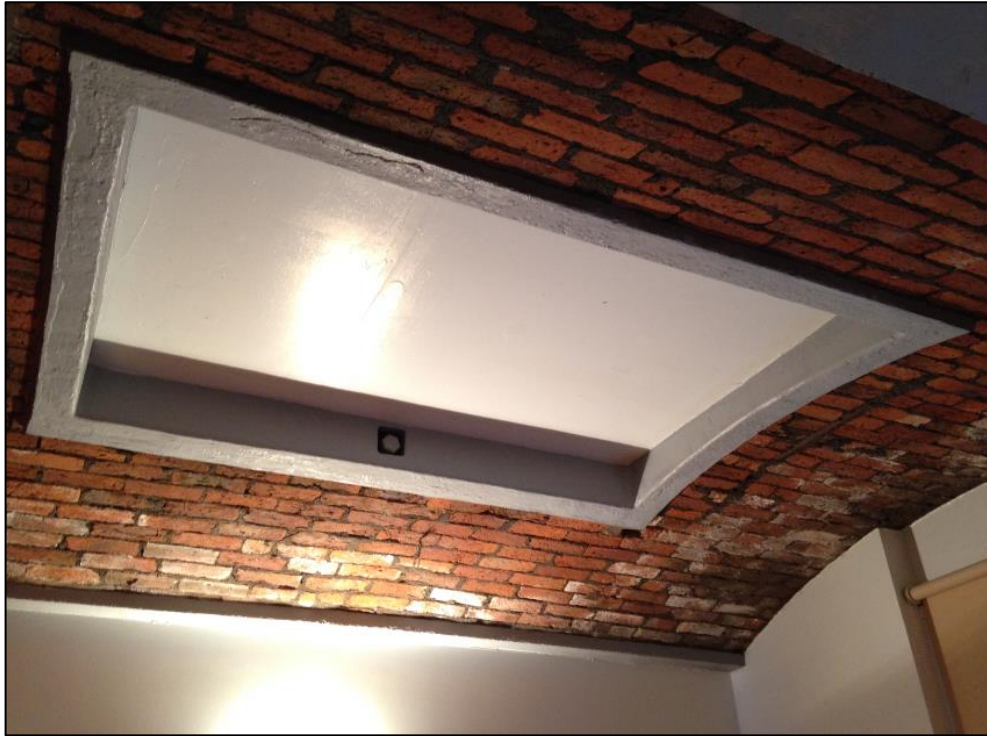
Figure 2.21: Blocked hoist bay
