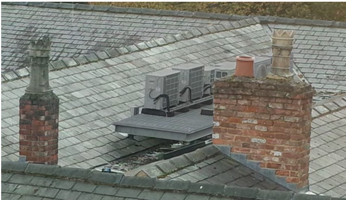
Enlarged view of air conditioning equipment taken from hotel bedroom with the equipment and platform structure painted in slate grey.
