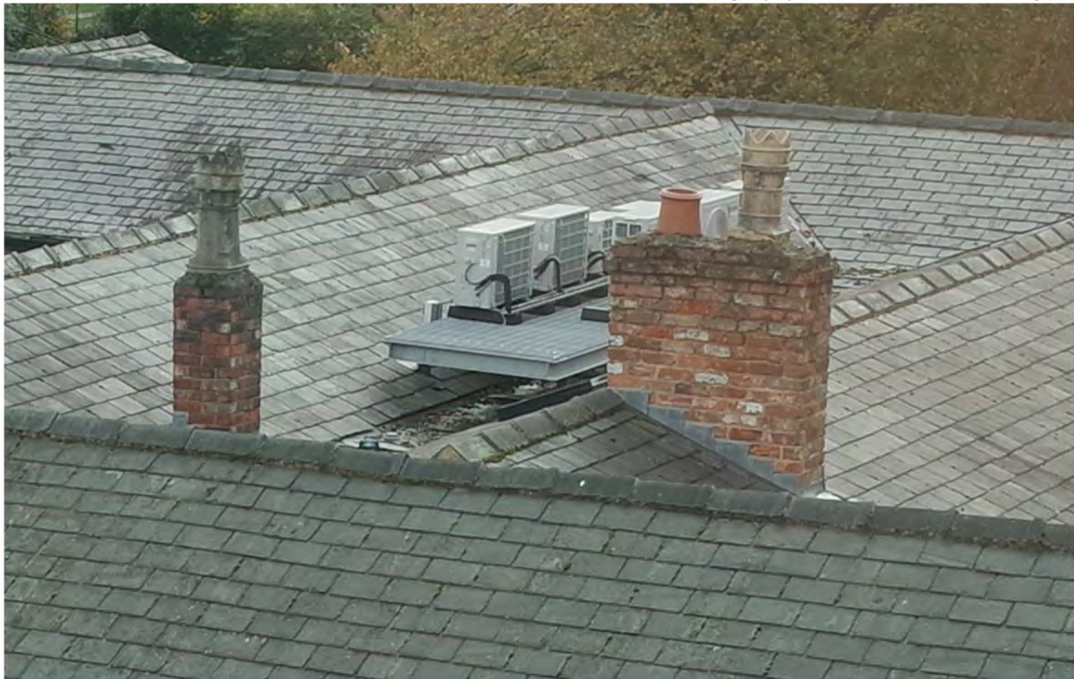
Enlarged view to show the new light grey finished equipment sitting on top of the galvanised steel platform.
