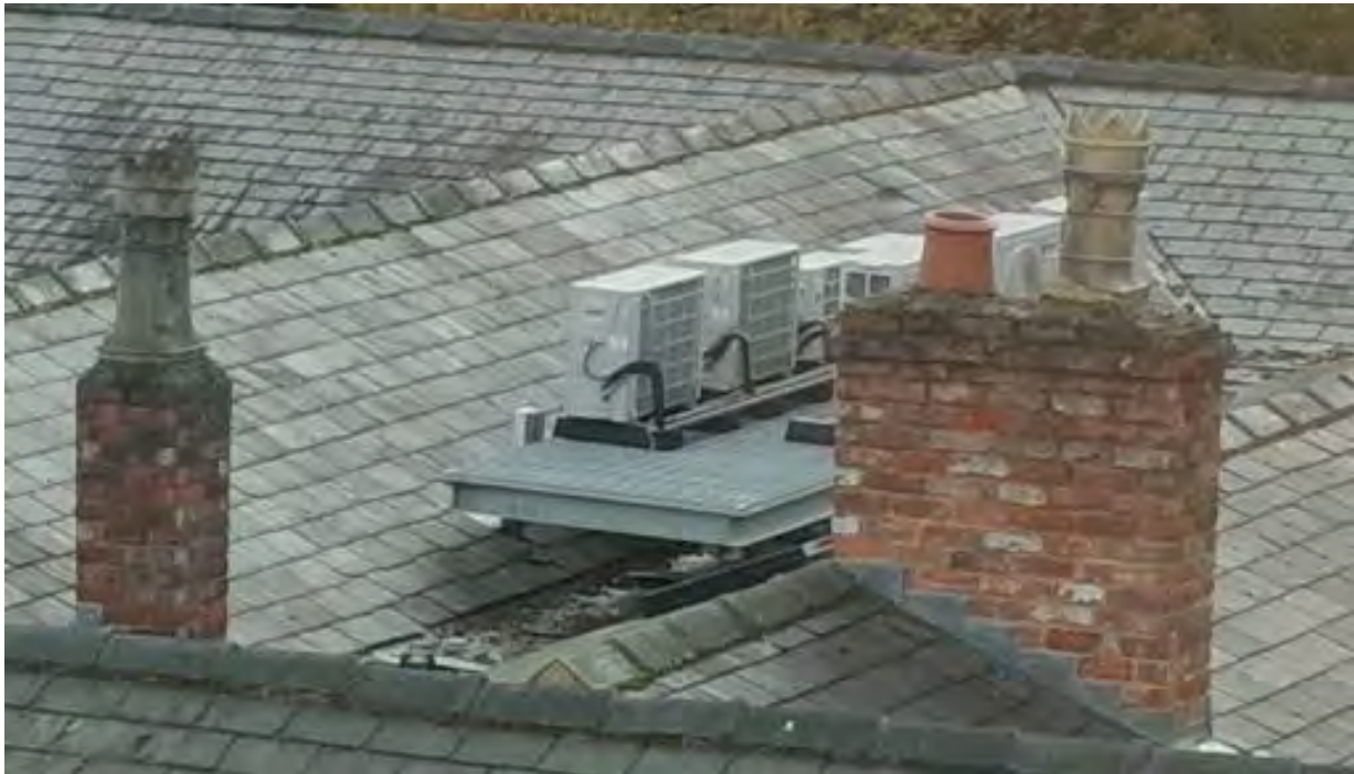
Enlarged view of air conditioning equipment taken from hotel bedroom.
