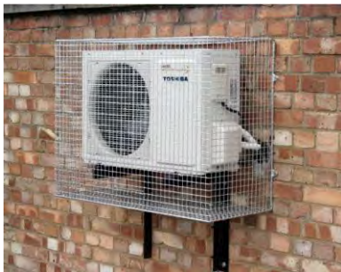
Typical example of wall mounted unit
