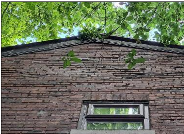
Photograph 6 showing gaps under the fascia on the south elevation
