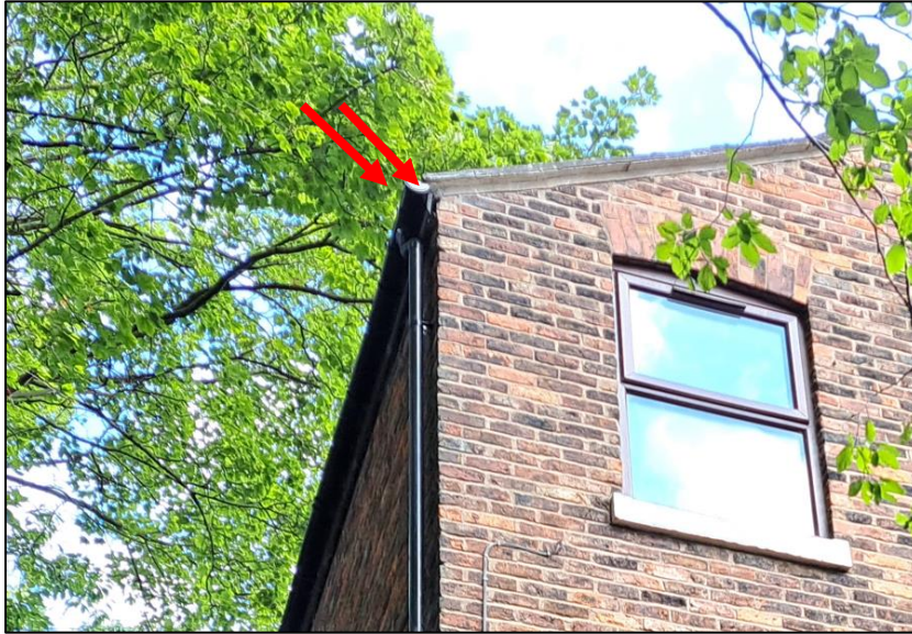
Photograph 8 showing the emergence locations on the southeastern elevation
