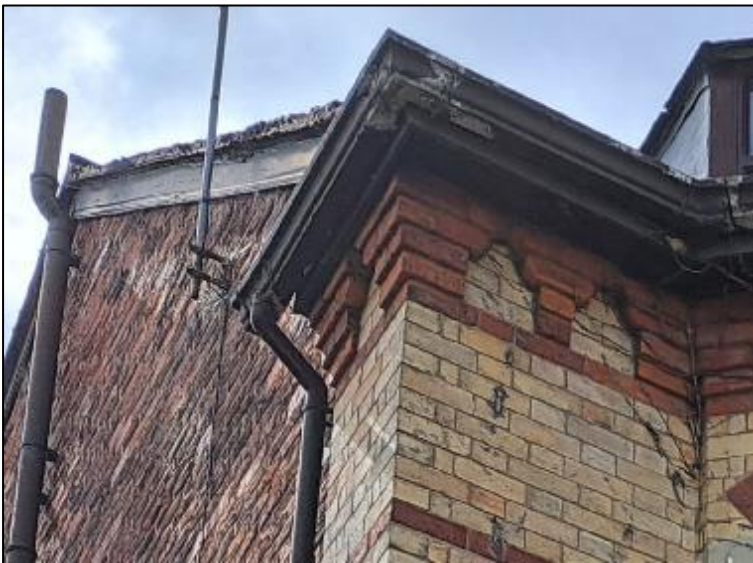
Photograph 5 showing gaps behind the wooden fascia on the north elevation
