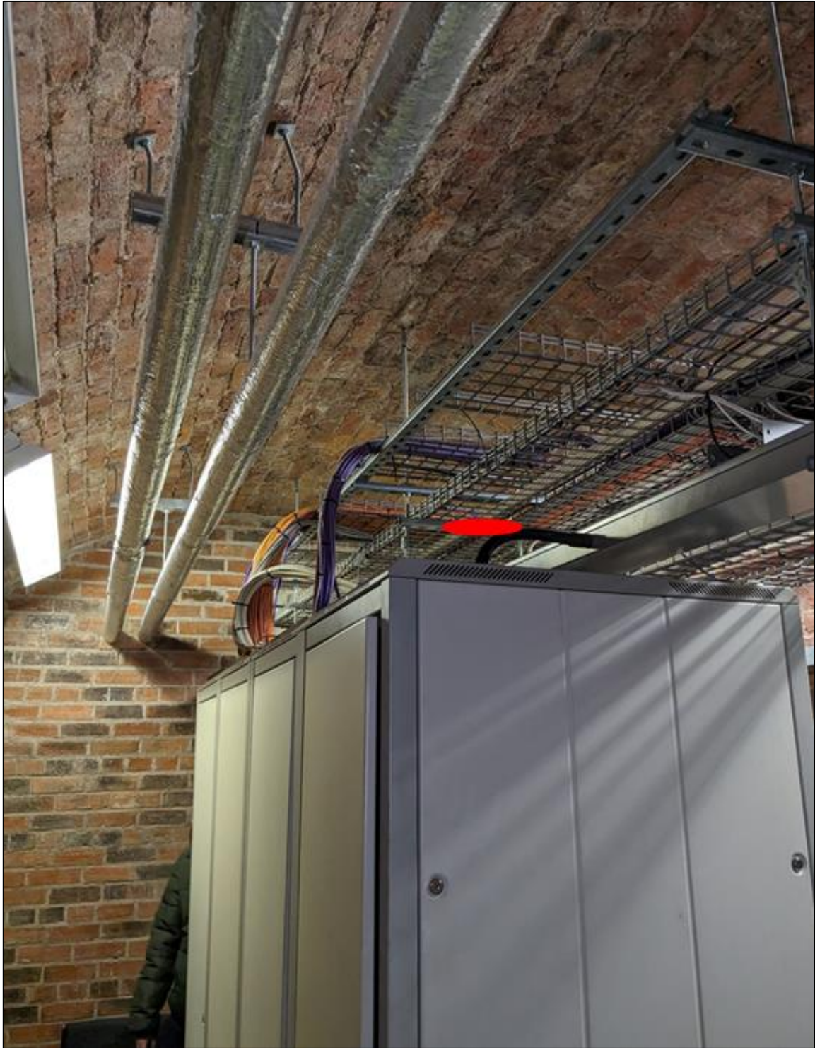
Appendix 1: The basement comms room is one of two in the building. LGAP4, as indicated by the red dot, is to be installed in the steel conduit tray pictured above the comms cabinet.
