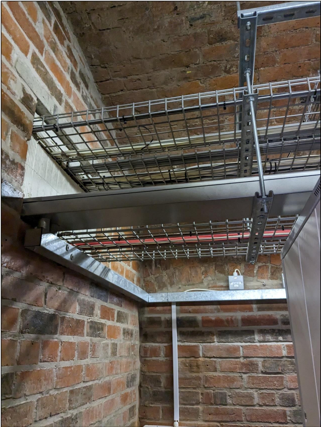
Appendix 2: Steel conduit tray and cable runs leaving the comms room to follow the route as mapped using a red line between LGAP4 and LGAP2.
