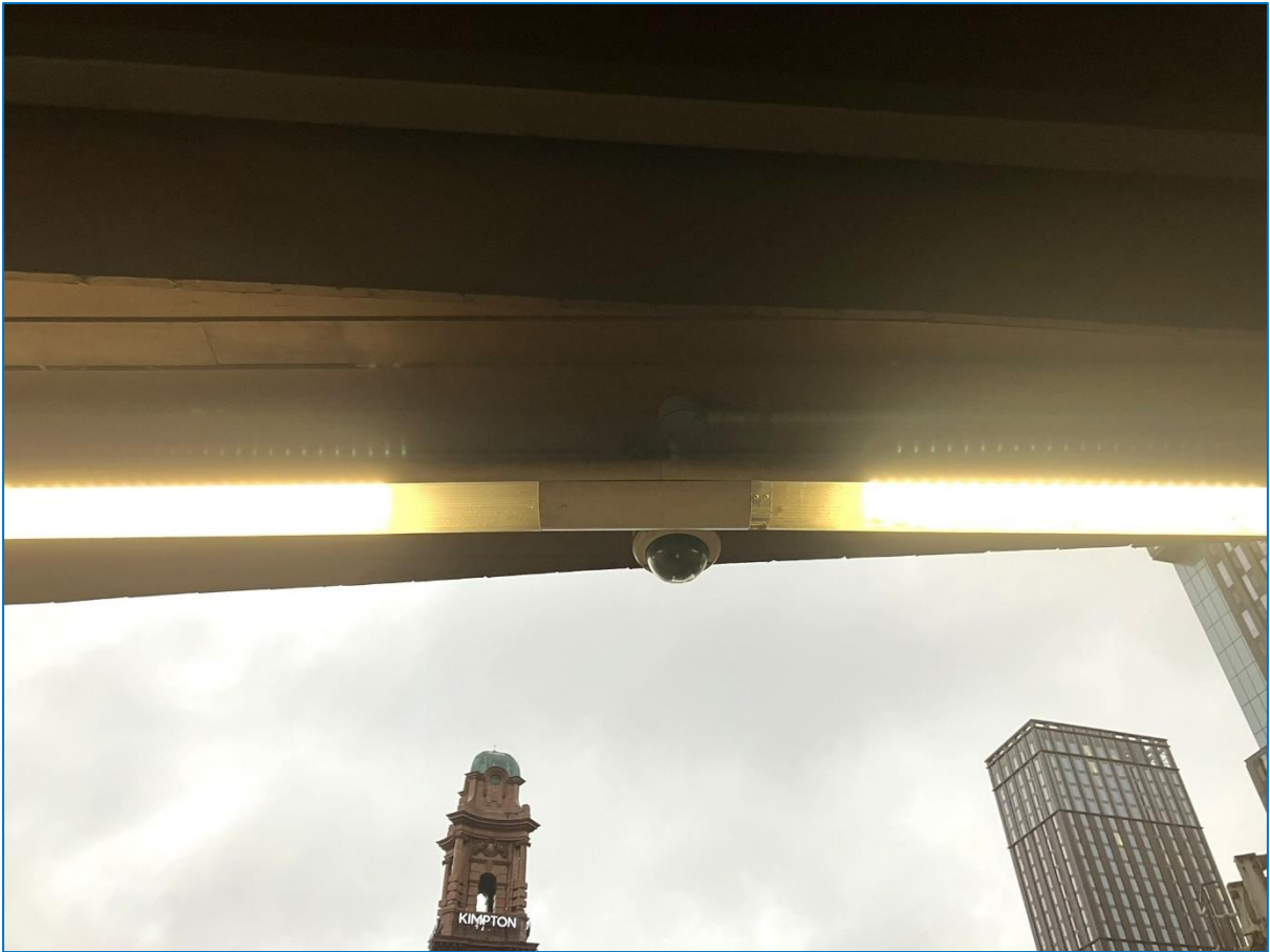
Figure 11 - Existing CCTV camera adjacent to strip lighting with ducting visible (taken from building side)
