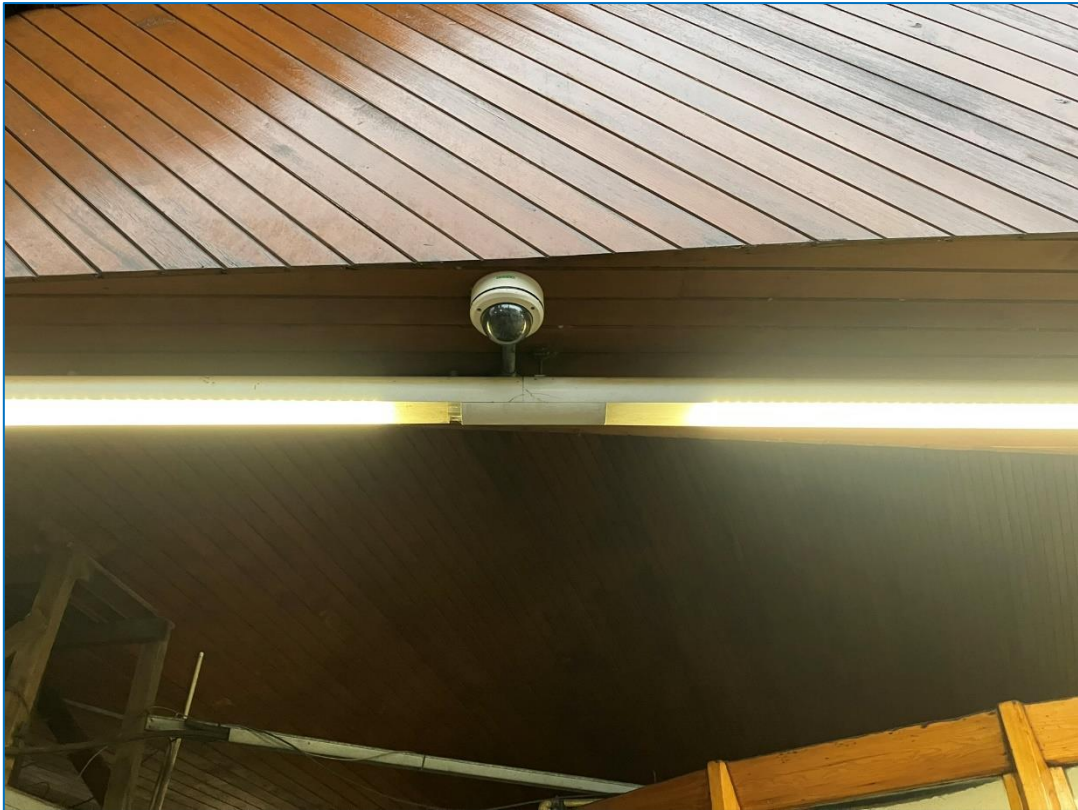
Figure 8 - Existing CCTV camera adjacent to strip lighting viewed from front.
