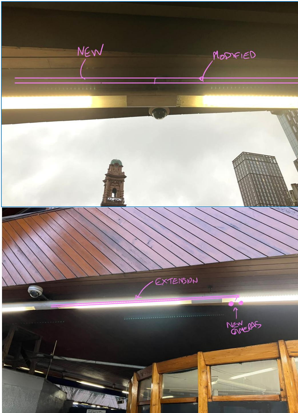
Figure 13 – Existing ducting fixed beneath/beside strip lighting – 3.2m extension of galvanised steel conduit
