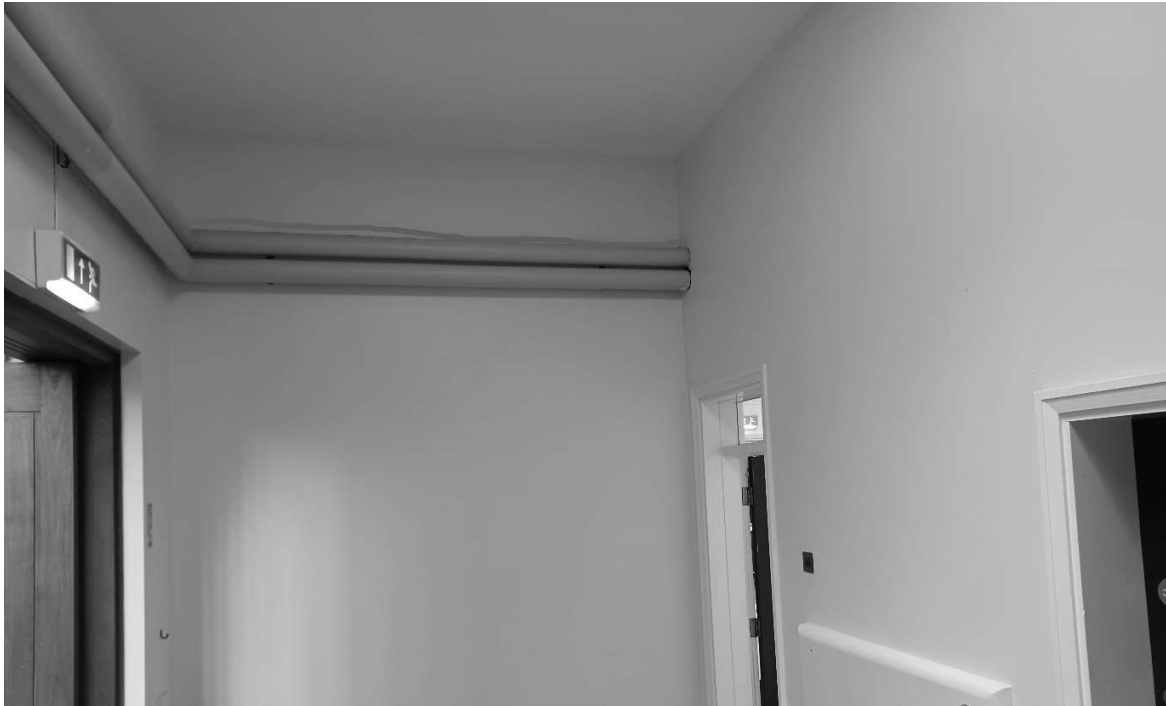
Cable Run 4 runs across Room B01–GF-011 from Hole 2 to Hole 4.
