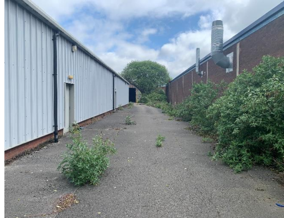
Photograph 6 – Hardstanding with buddleia growing through
