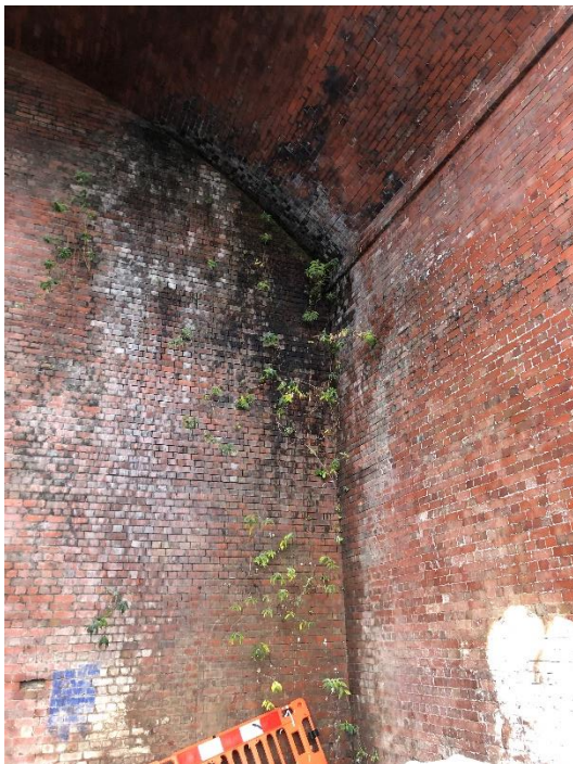
Figure 2-11 Damp areas beneath the arches in the north of the site due to open pipes draining the trackway above.
