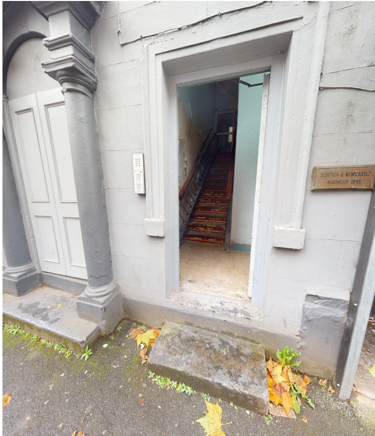
Existing ground floor entrances to the hotel involve a rise of over 250mm.
