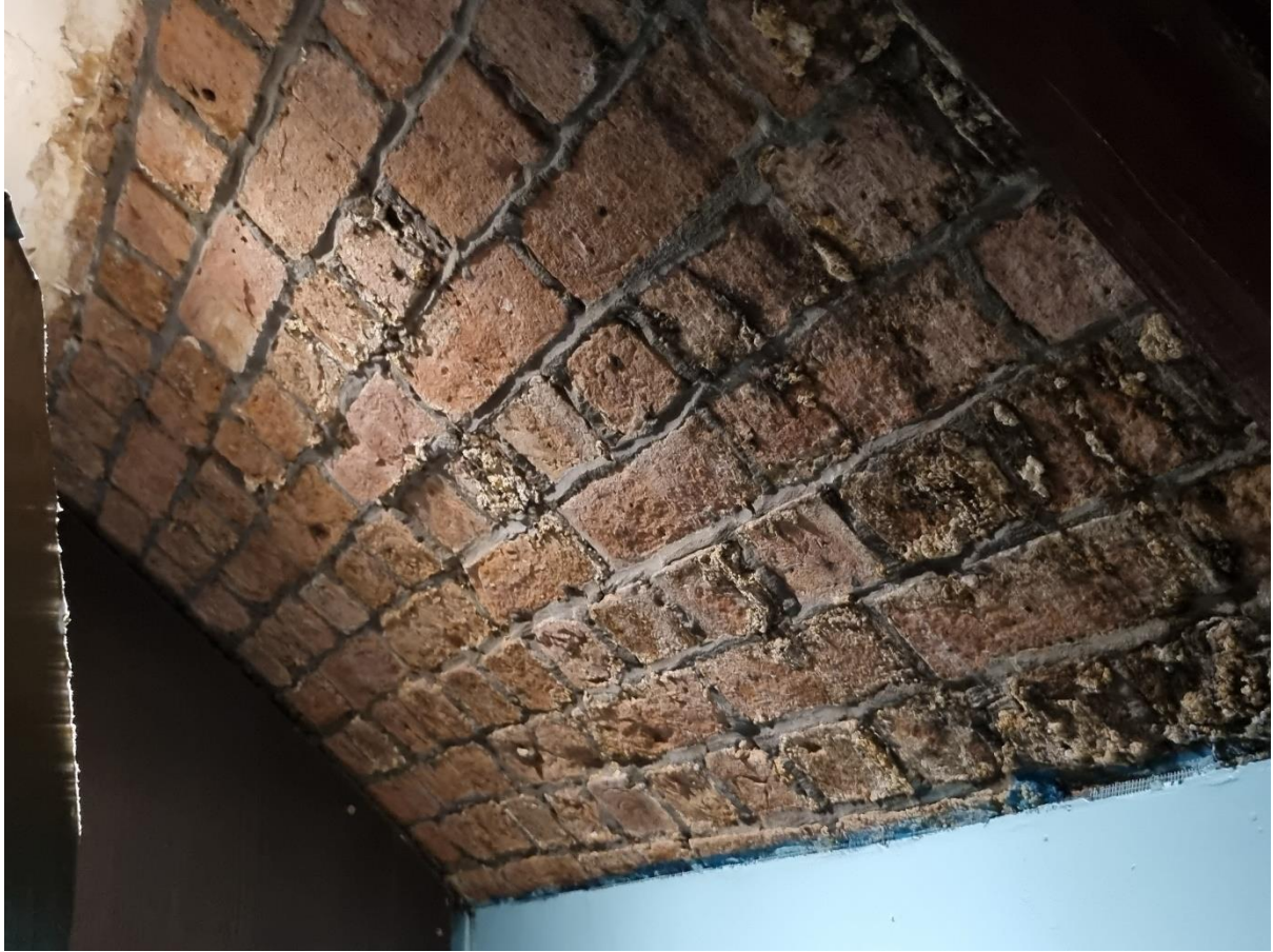
Typical water ingress to soffit
