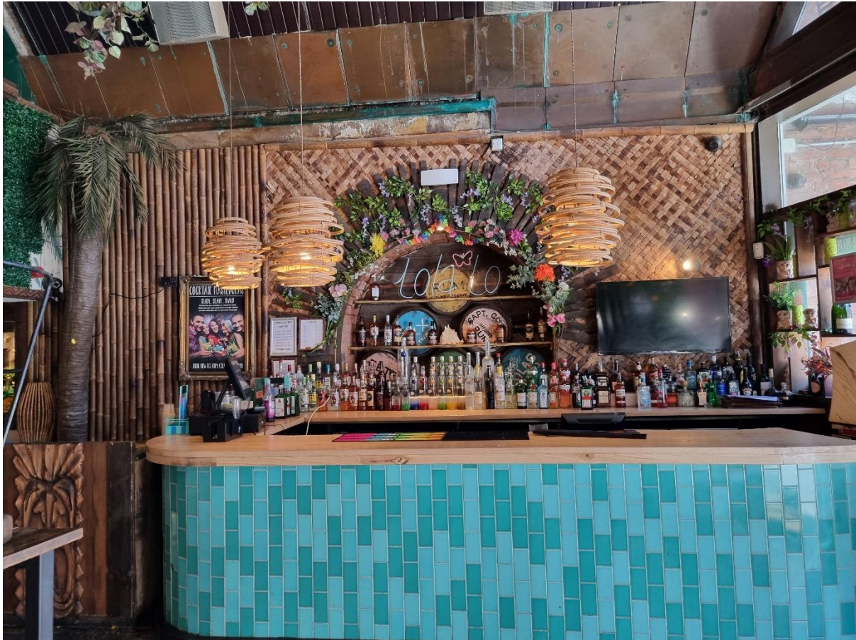
Original copper panels, impacted by water.
