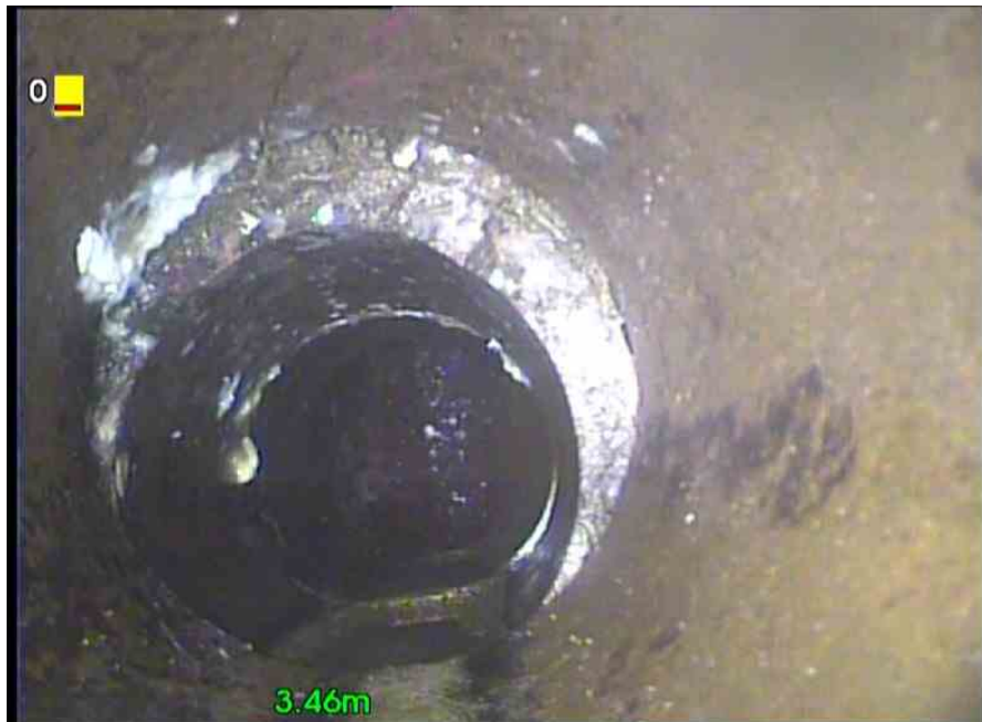
, 00:01:17, 3.46 m Joint displaced, medium
