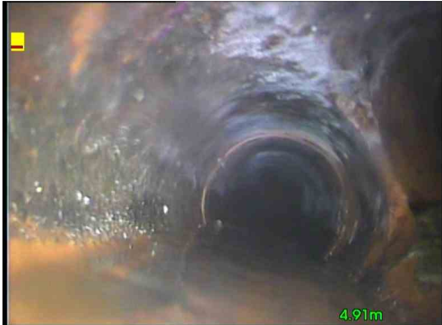
, 00:01:10, 6.49 m Crack, circumferential from 12 o'clock to 4 o'clock
