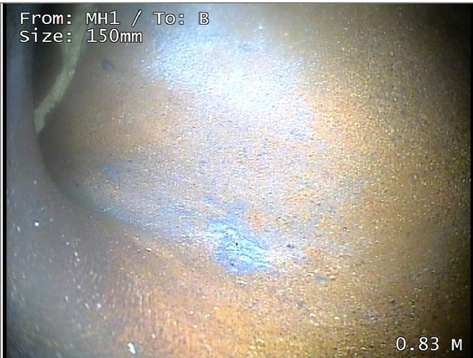
Line of drain/sewer deviates up
