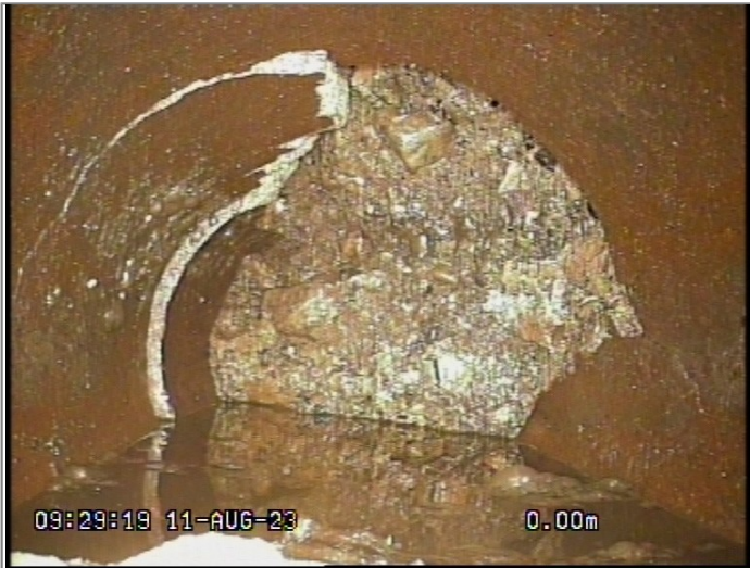
Start node type, manhole, reference MH3
