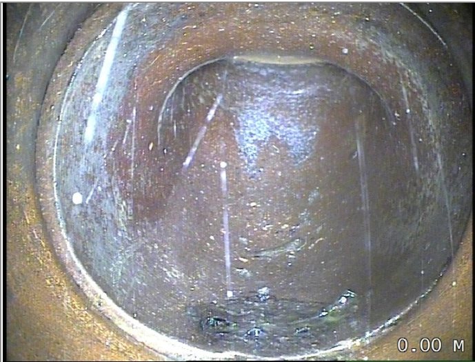
Start node type, manhole, reference MH6
