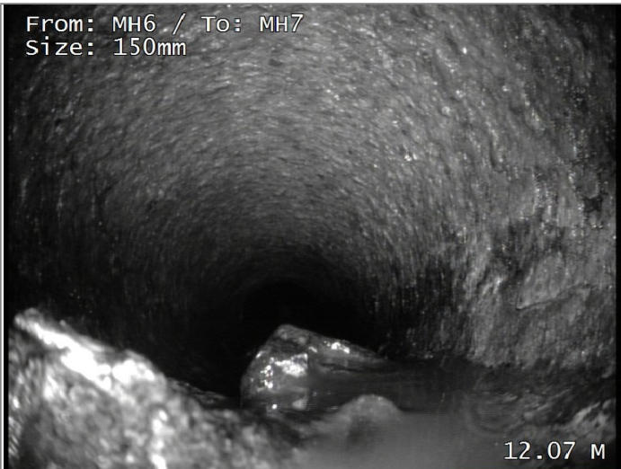
Settled deposits coarse 25% cross-sectional area loss
