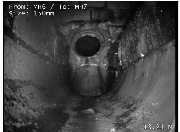
Finish node type, manhole, reference MH7
