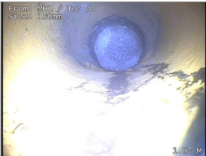
Line of drain/sewer deviates up
