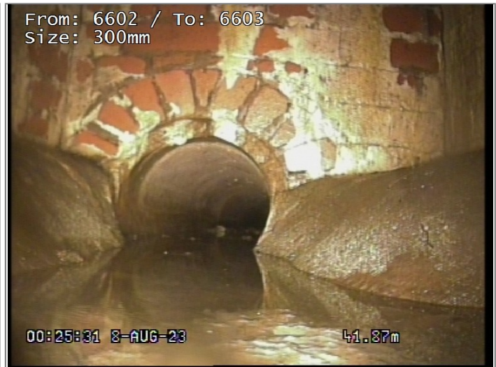
Settled deposits coarse 10% cross-sectional area loss, Finished
