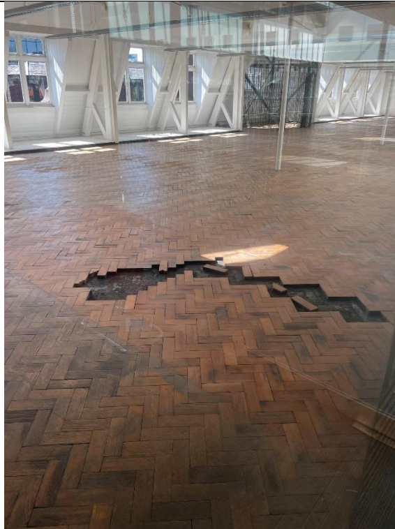
Figure 55: Fifth floor. Evidence of damage to original parquet floor.
