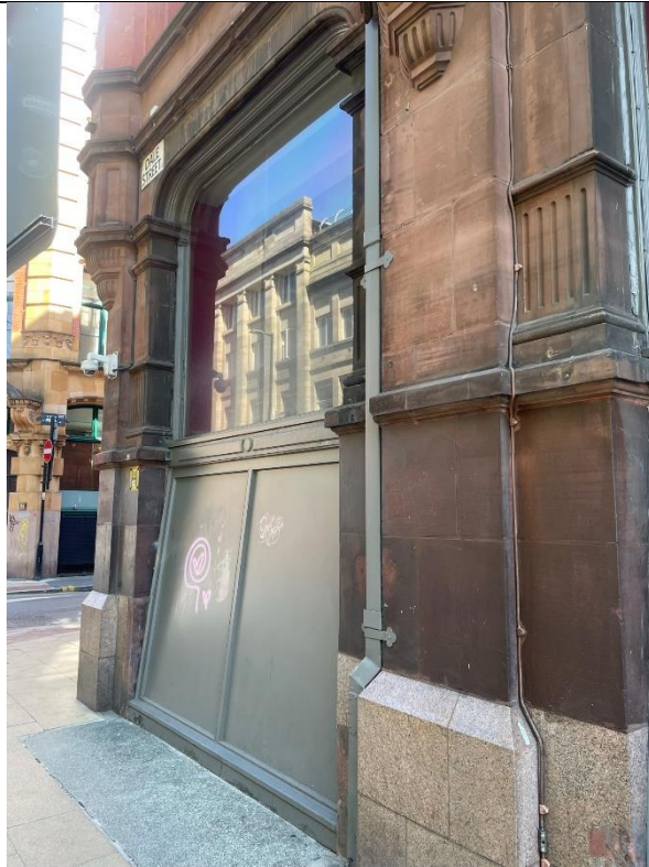
Figure 30: Dale Street elevation. Basement windows overcovered with film / opaque paint. Original glazing bars have been removed.
