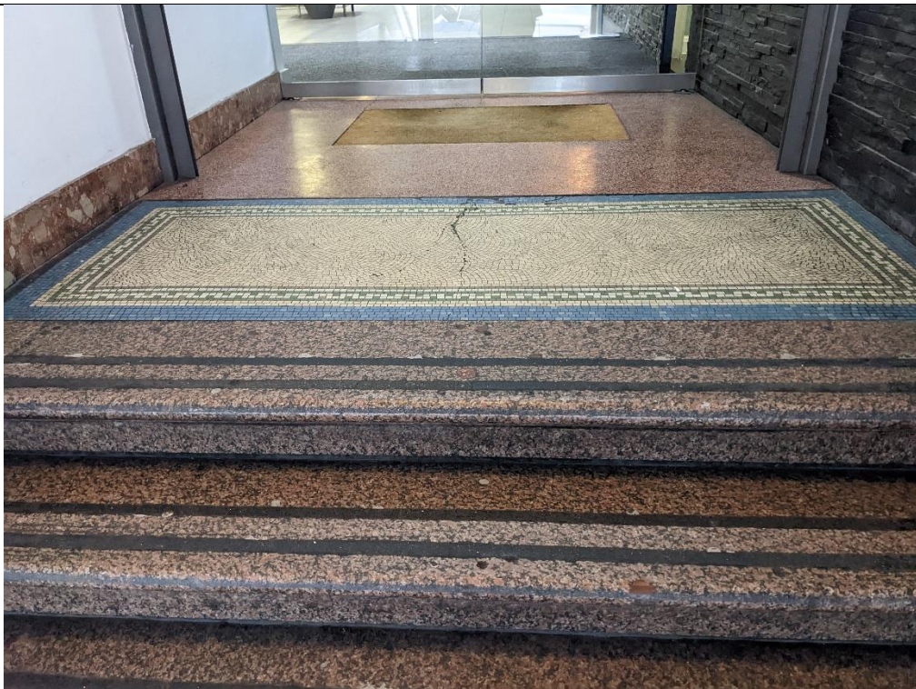
Figure 35: Main entrance, Dale Street. Original mosaic / terrazzo entrance stair. Evidence of cracking and in need of general maintenance / repair. Modern walls and glazing to entrance lobby.
