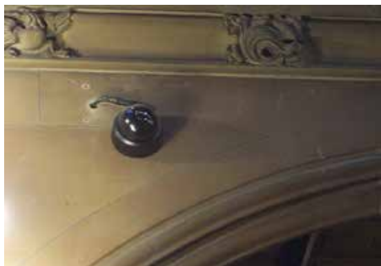
Fig 30. Inappropriate installation of CCTV camera
