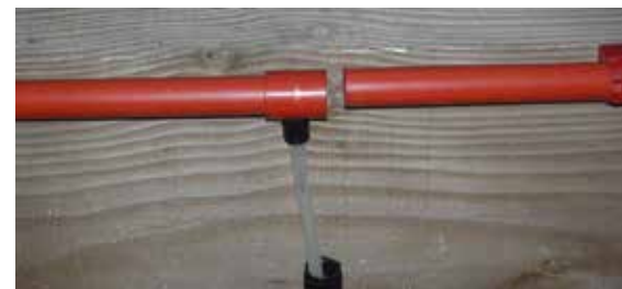
Fig 27. VESDA system within main roof void
