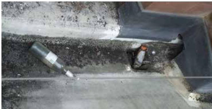
Fig 26. Example of inappropriate building maintenance
