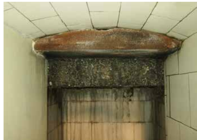
Fig 26. Water ingress to pavement light infills
