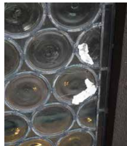
Fig 27. Example of inappropriate building repair
