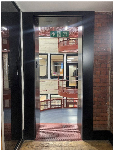
Figure 6: Looking SW from east unit (former Berghaus unit, 3 rd floor) towards central atrium. Note, there is no fire door to this entrance.
