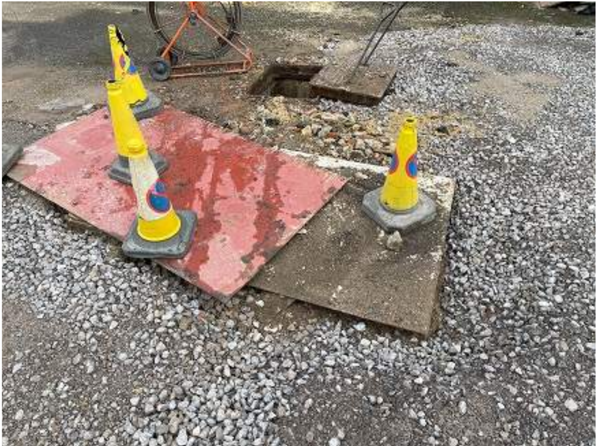
INTERCEPTOR 1 UNDER PLATES
