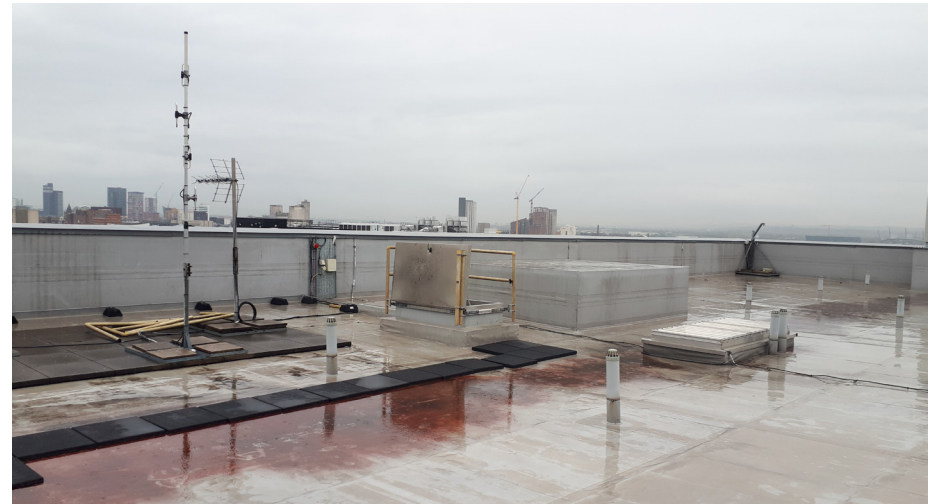
Figure 6 - Noticeable standing water on the roof
