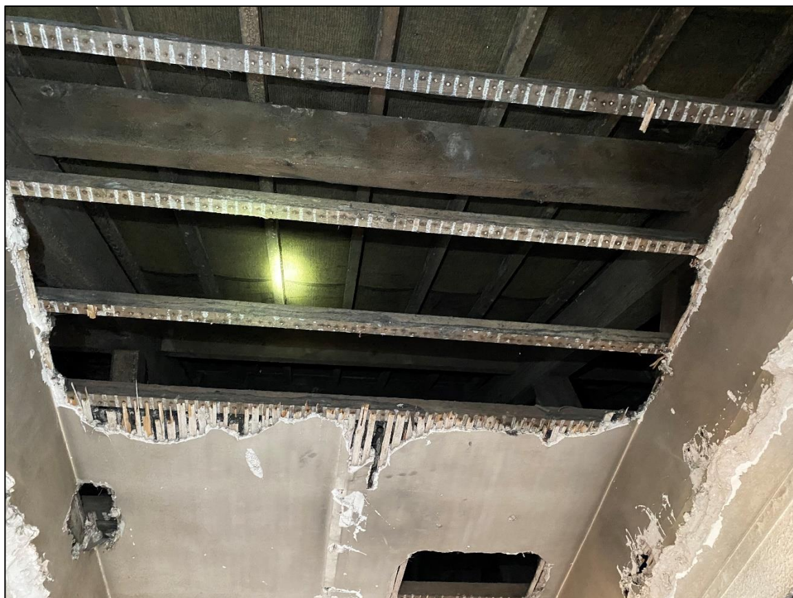
Plate 5 – Open/collapsed nature of much of the loft
