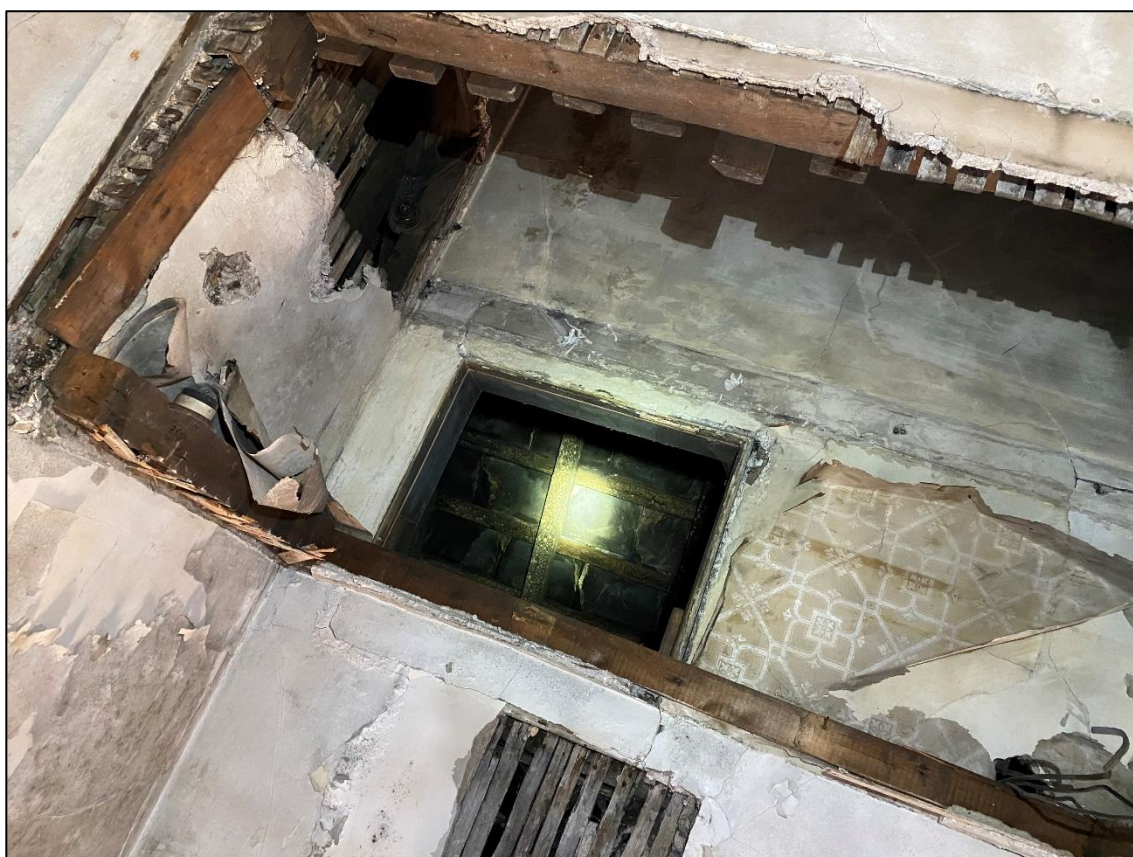
Plate 4 – Absence of underlining in areas of the roof
