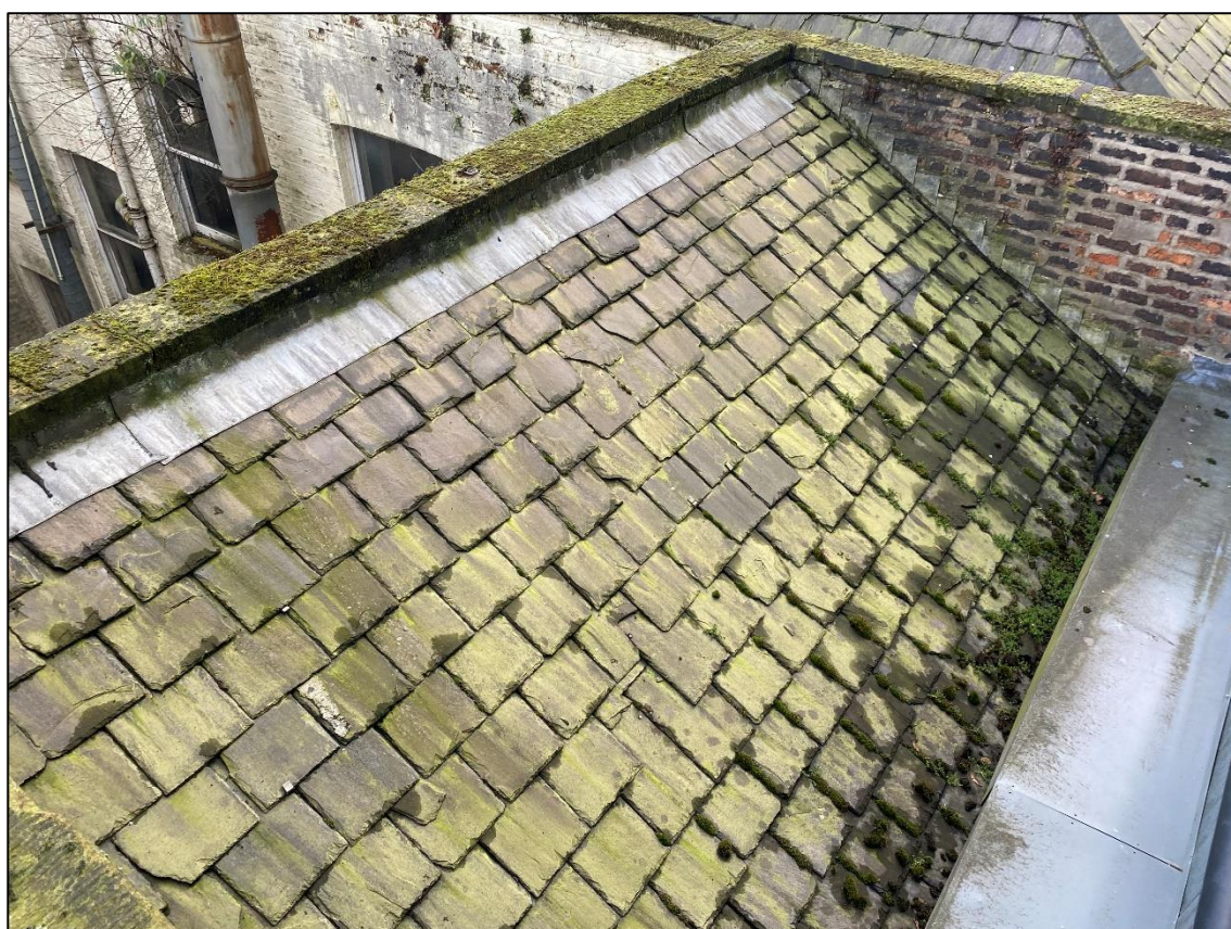
Plate 8 – Numerous gaps beneath slipped/lifted slates on the roof pitches accessed
