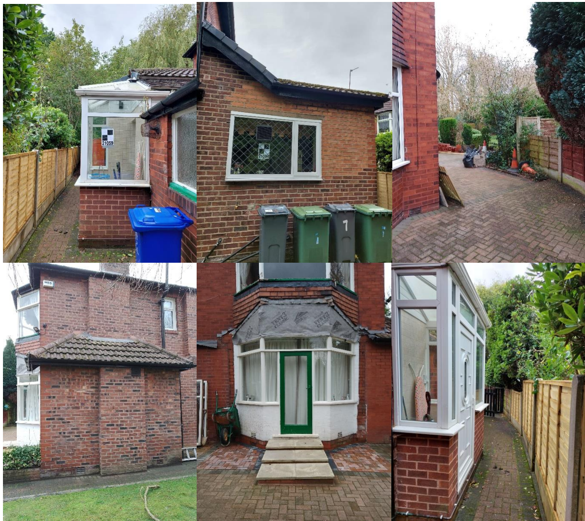
Various photos showing the existing extensions and modifications which are either of poor quality or not in-keeping with the style of the house. These include blocked up windows, peeling paint and mis-match brickwork.
