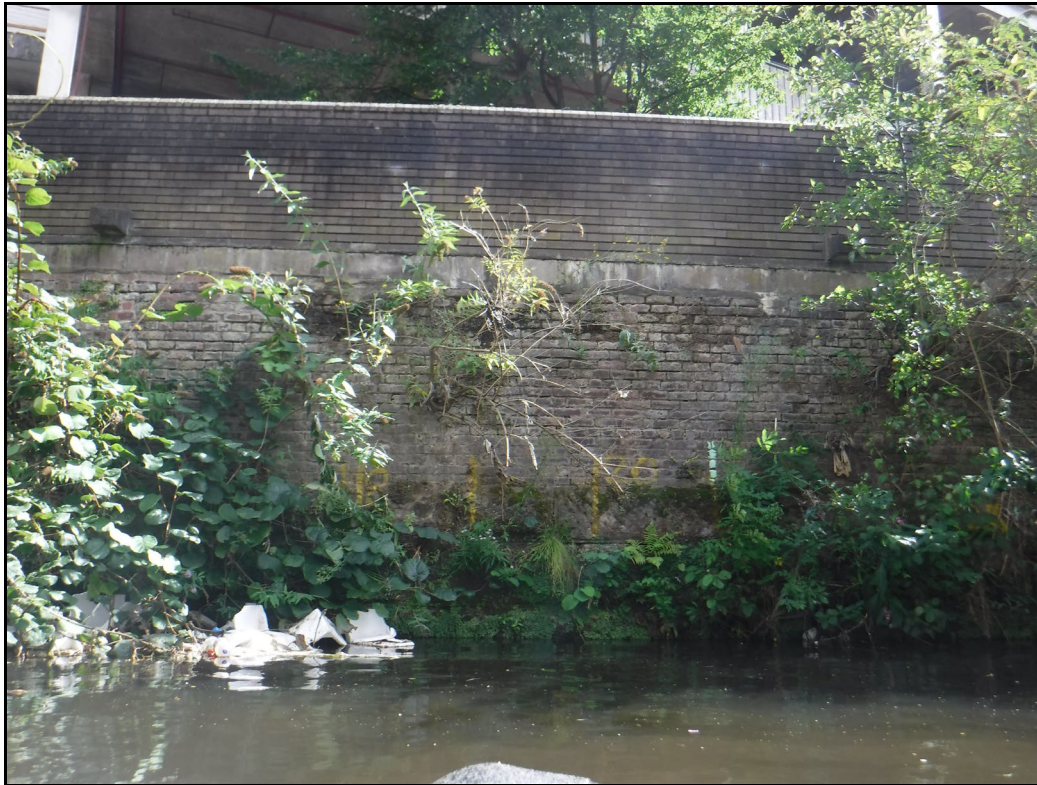
Above:- General view of Ch120m showing condition of wall
