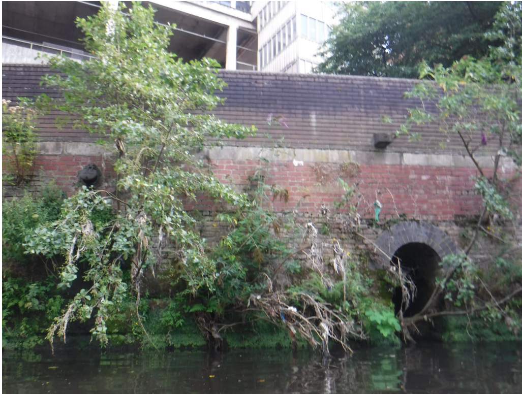
Above:- Ch145m, showing vegetation growth and culvert entrance
