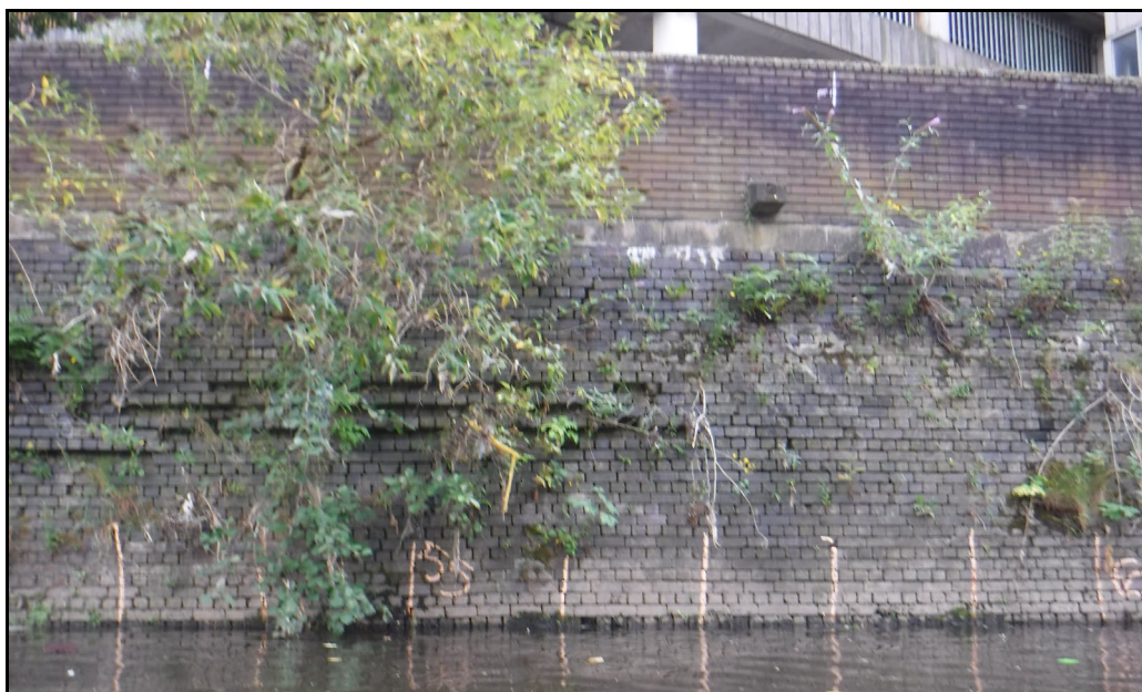
Above :- Ch 55m, displaying displacement of brick courses due to tree and vegetation growth.
