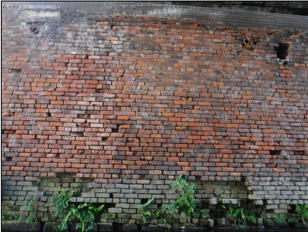
Above:- Ch 175m, showing condition of displaced brickwork
