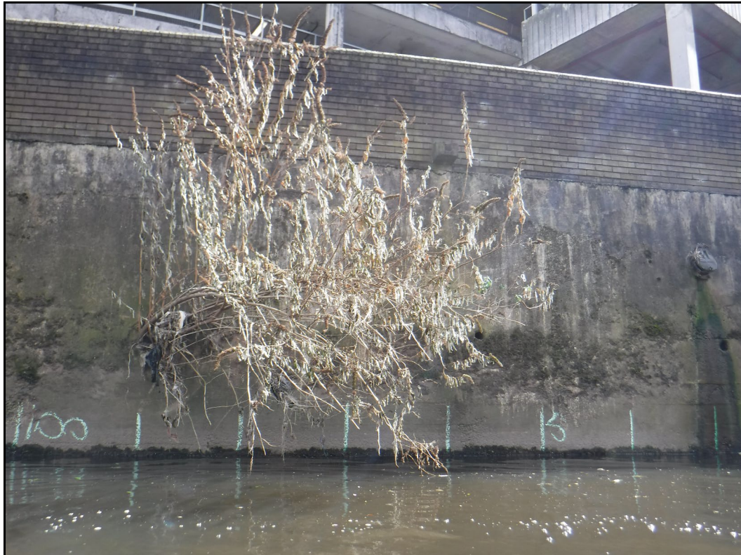
Above:- General view around Ch102m showing vegetation growth through concrete wall
