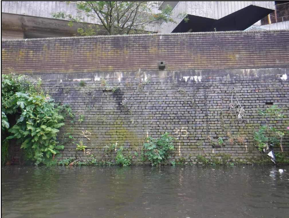
Above:- General view of wall at Ch 35m. Open joints and vegetation growth
