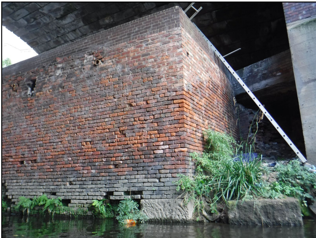
Above:- Ch 182m, showing condition of displaced brickwork. End of survey.
