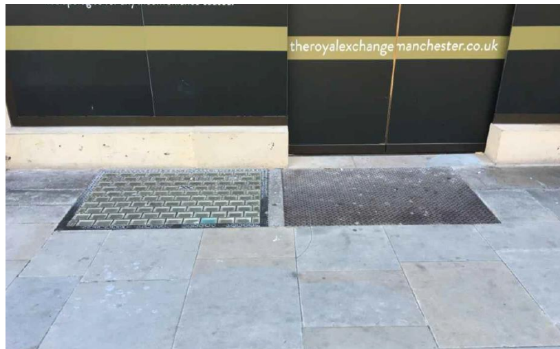
(Figure 3: An example of the proposed replacement light alongside a steel plate fitted over, as is the case for some of the locations. Please current condition and replacement locations fully outlined in accompanying plan titled: "PAVEMENT_LIGHTS_WITH_PHOTOGRAPHS".)
