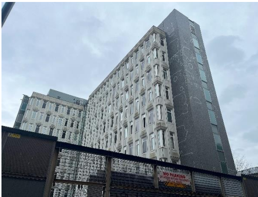
Figure 2.2 Chatsworth House as seen from Back Piccadilly, note the sections of failing tiling.
