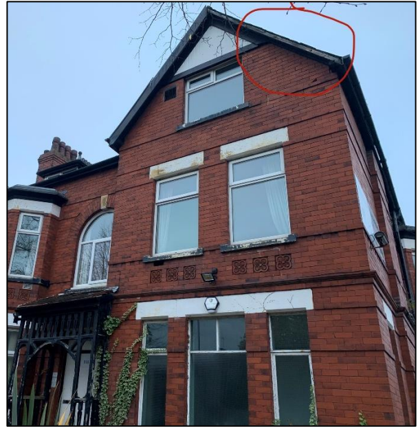
Missing barge board
