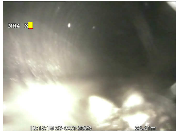
Photo: 74_6a, 00:00:00 24.4m, Debris silt, 10 % cross-sectional area loss, Start
