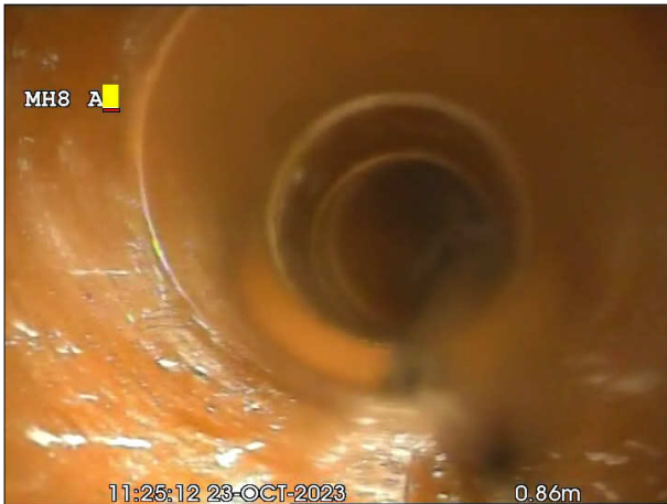
Photo: 17_4a, 00:00:00 0.3m, Junction at 06 o'clock, dia 150 mm, Remark: Back drop
