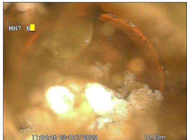
Photo: 98_7a, 00:00:00 10.9m, Debris, 30 % cross-sectional area loss
