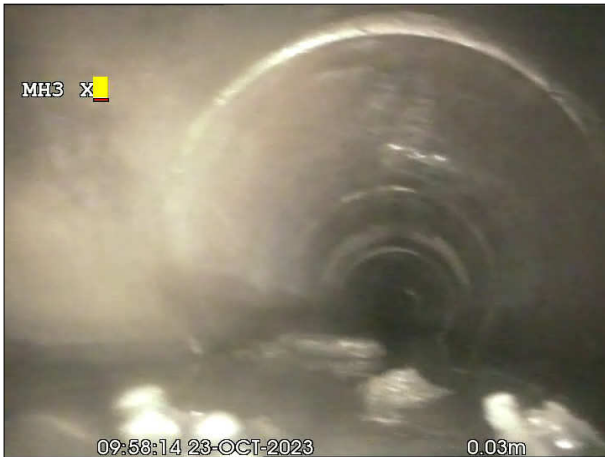
Photo: 45_4a, 00:00:00 0m, Debris silt, 10 % cross-sectional area loss, Start
