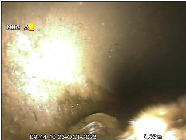
Photo: 30_4a, 00:00:00 1m, Debris, 20 % cross-sectional area loss
