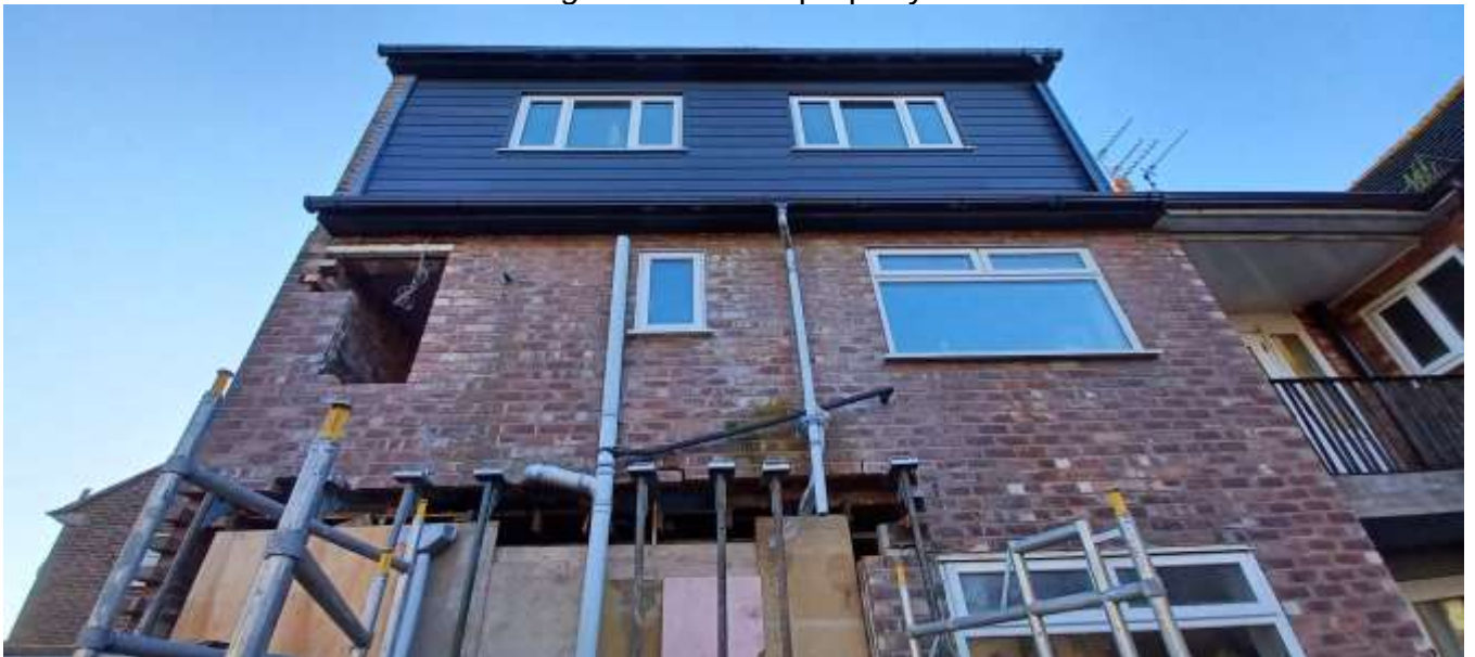
Figure 3. Unauthorised third storey rear extension.
