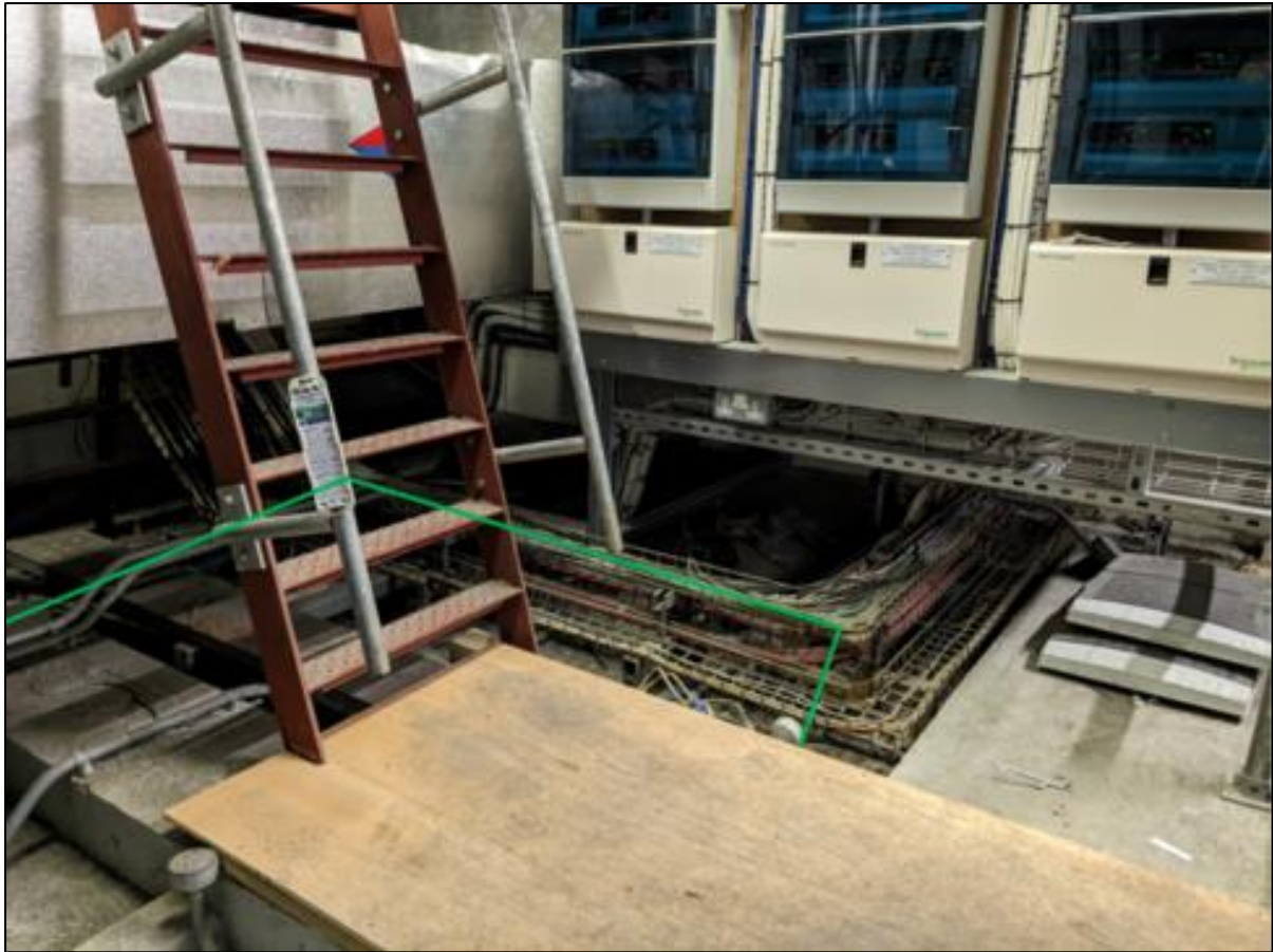
Appendix 52: The cable run above, pictured in green, enters 003 Plant Room via 006 Service Riser pictured in Appendix 55. From the riser the cable follows the steel conduit tray pictured above to an existing drill used to wire a lightbulb (pictured in Appendix 58) and to a cavity which provides access to 021A Services.
