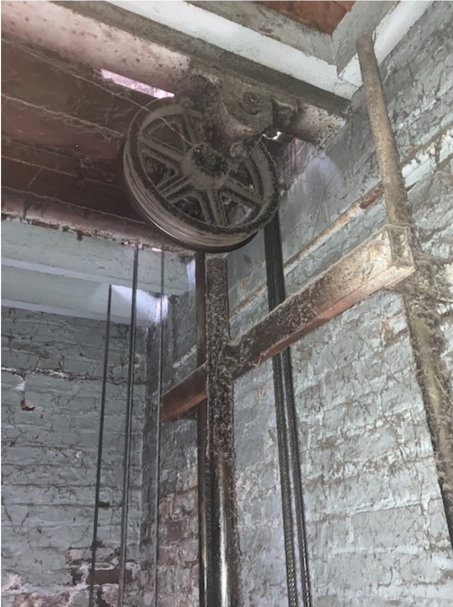
ITEM G7 Lift pulley at head of shaft
