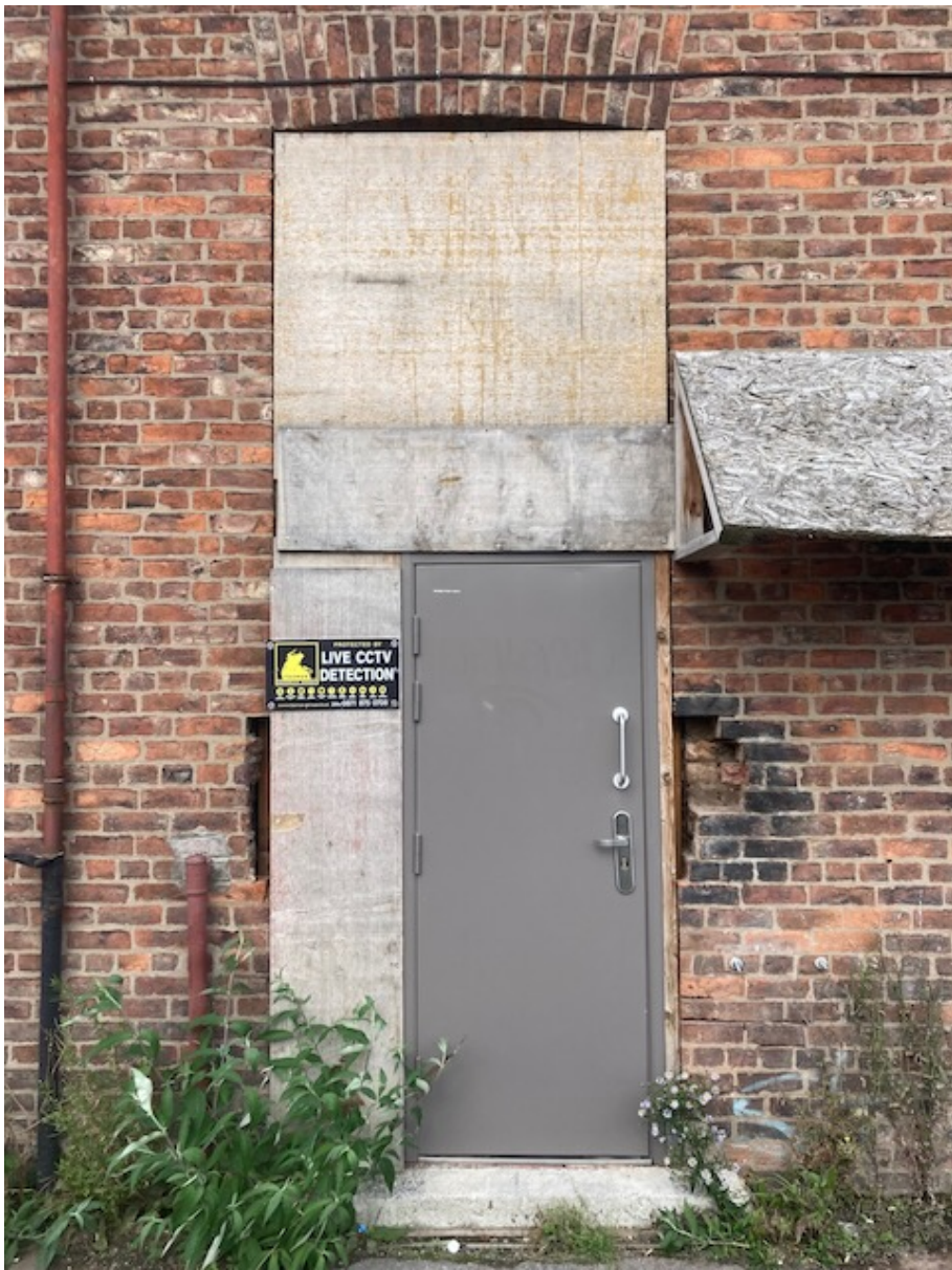
ITEM 08 Timber doors and damaged brick reveals to Baird Street opening
