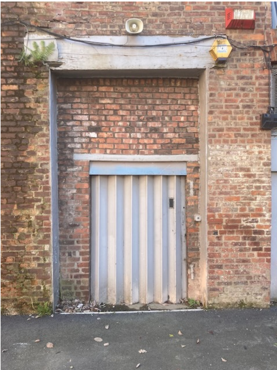
ITEM G7 External lift doors at ground floor
