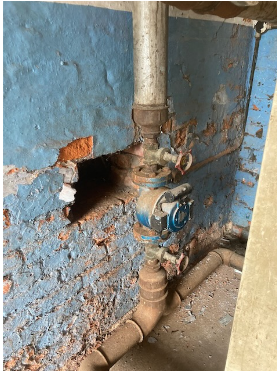
ITEM G9 Valve arrangement alongside boiler
