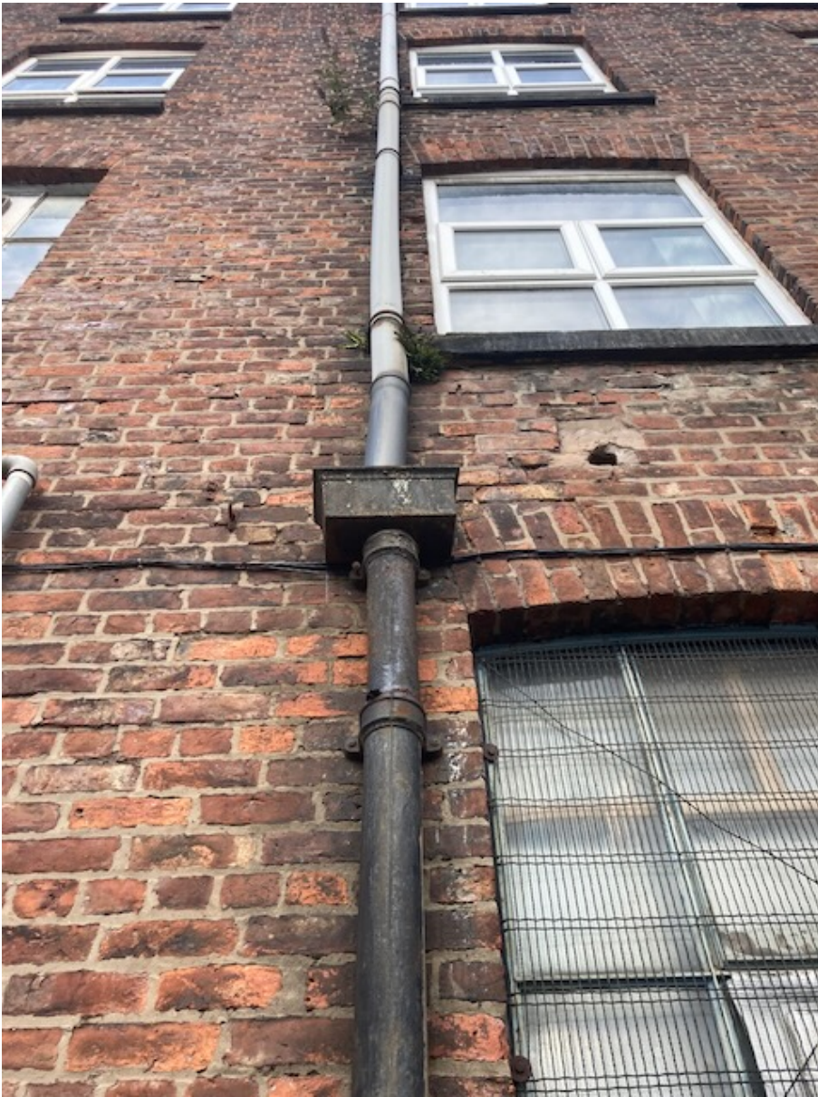
ITEM G14 Part plastic part cast iron hopper head and pipework to Baird Street
