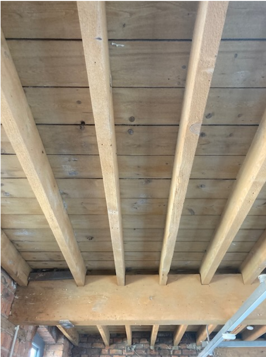
ITEM G3 / G4 Exposed joists and timber boards at 3rd floor
