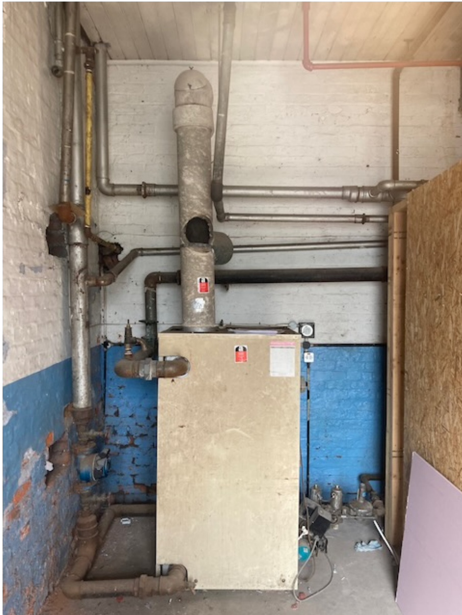
ITEM G9 Boiler installation at ground floor
