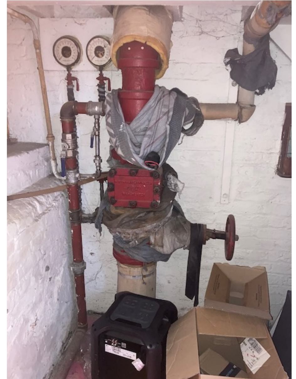
ITEM G8 Sprinkler valves within North East Stair
