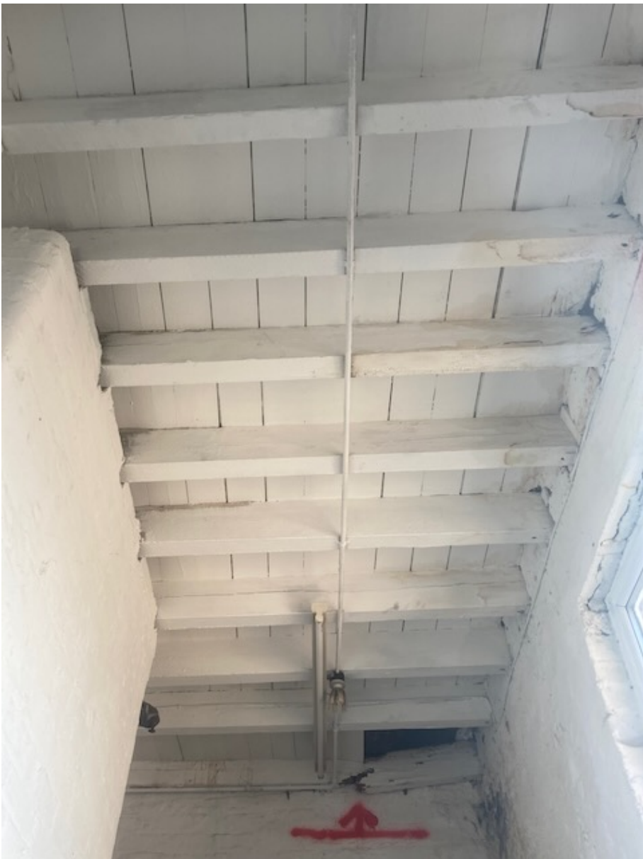
ITEM G11 Timber joists and soffit to top floor of north east stair
