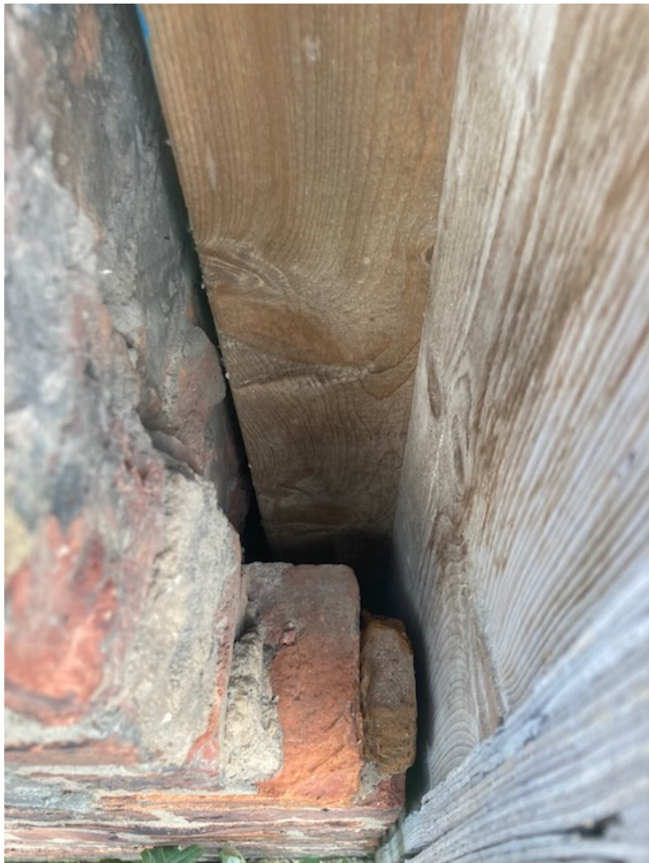
ITEM 08 Damaged brick reveals to Baird Street opening
