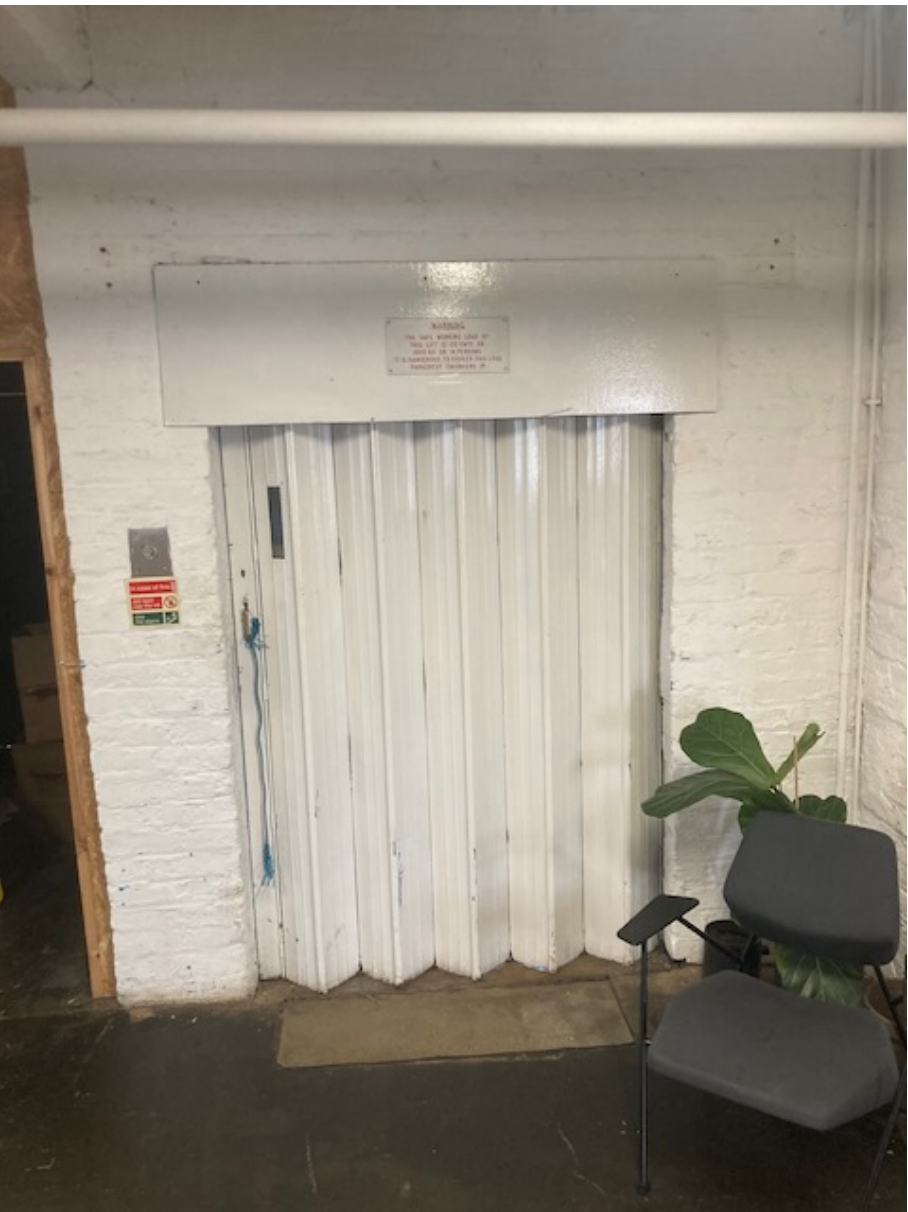
ITEM G7 Internal lift doors at 1st floor
