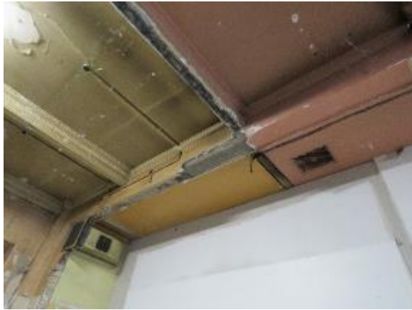
Figure 56: View of ceiling ventilation ductwork.
