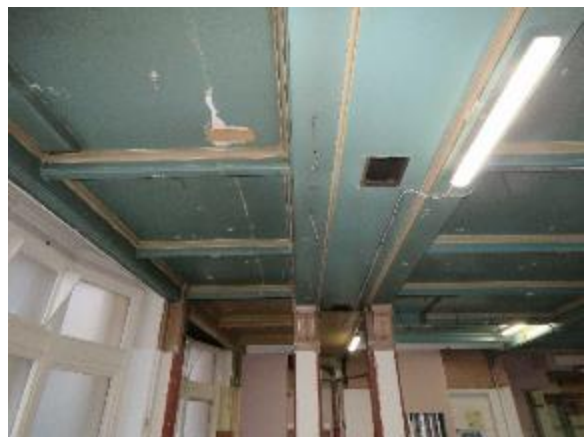
Figure 61: View of ceiling with ventilation ductwork integrated with structural design.
