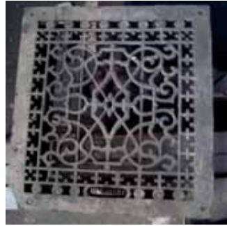
Photo 39 - EB.6F.01- Stray vent cover on 6 th floor
