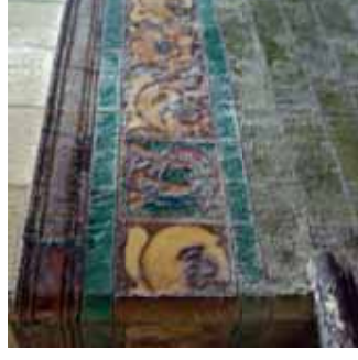
Photo 18 – Tiles crazing on lower levels
