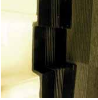
Photo 55. HB.1F.27- Early skirting
