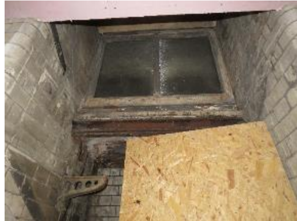
Figure 27: One of the surviving lower ground floor windows currently boarded over.
