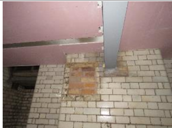
Figure 29: One of the original hot air ventilation openings now blocked up.
