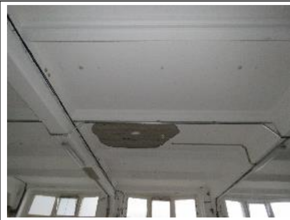
Figure 68: View of ceiling with section of failed plaster.
