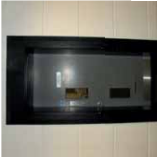
Photo 63. HB.3F.15 – Typical architrave found on 3 rd floor, disfigured by later interventions.
