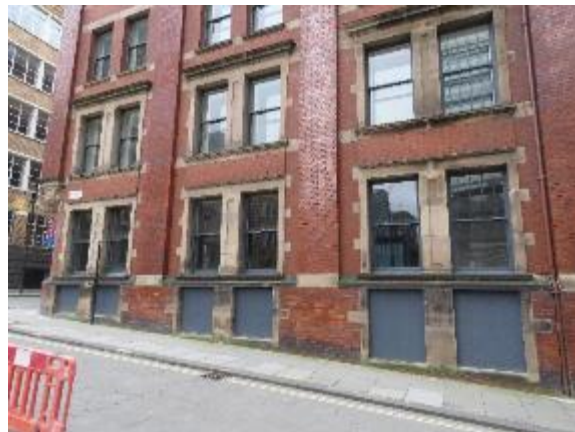
Figure 11: View of the three window bays of E Block from Hanover Street with basement windows boarded over.
