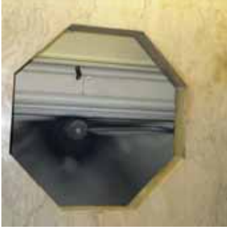
Photo 45. HB.GF.21- Early ceiling covering original ceiling
