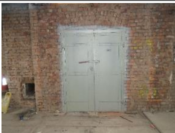
Figure 38: Surviving steel riser doors and exposed brickwork.
