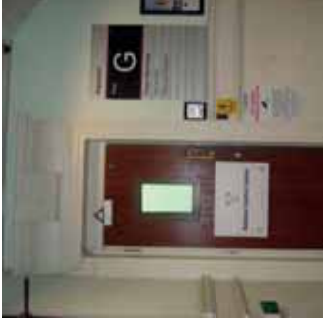
Photo 30. HB.GF.19- Original opening and architrave
