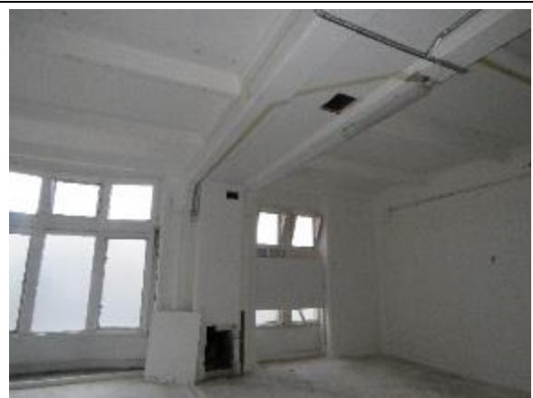
Figure 69: General view of ceiling ductwork and structural beams.
