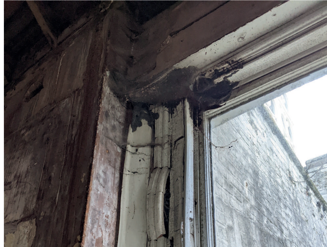
Typical window frame condition. Refer to separate report for further images.
