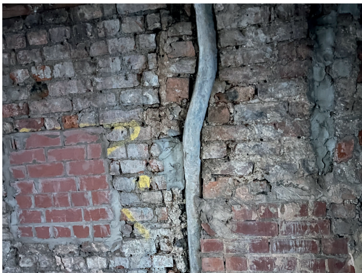
Lead RWP internally in poor condition- to be replaced with cast iron.
