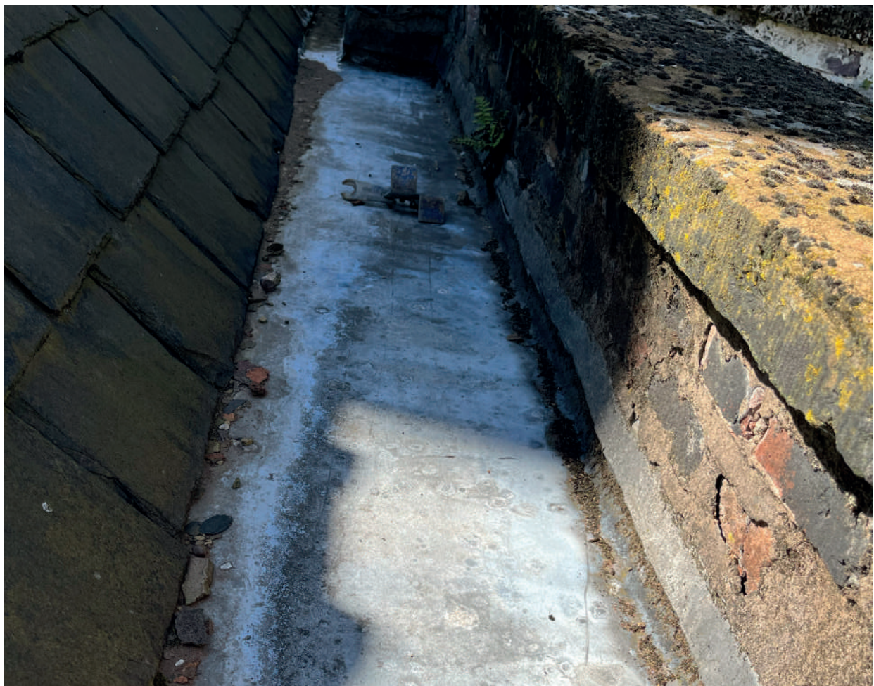
Slates installed incorrectly- resting on gutter sole. Flashing to be renewed.
