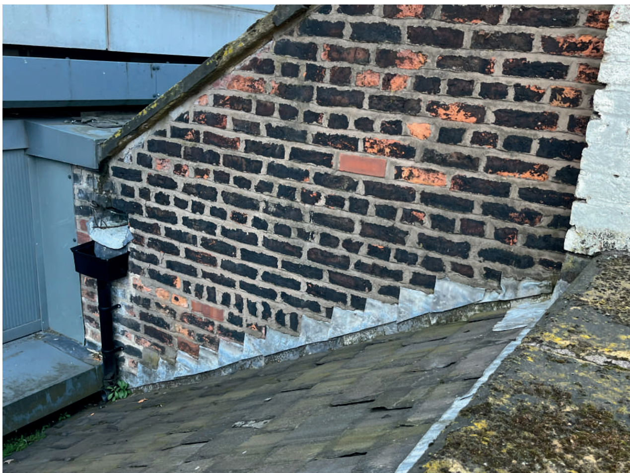
Flashing renewal required. Plastic RWP to be replaced.
