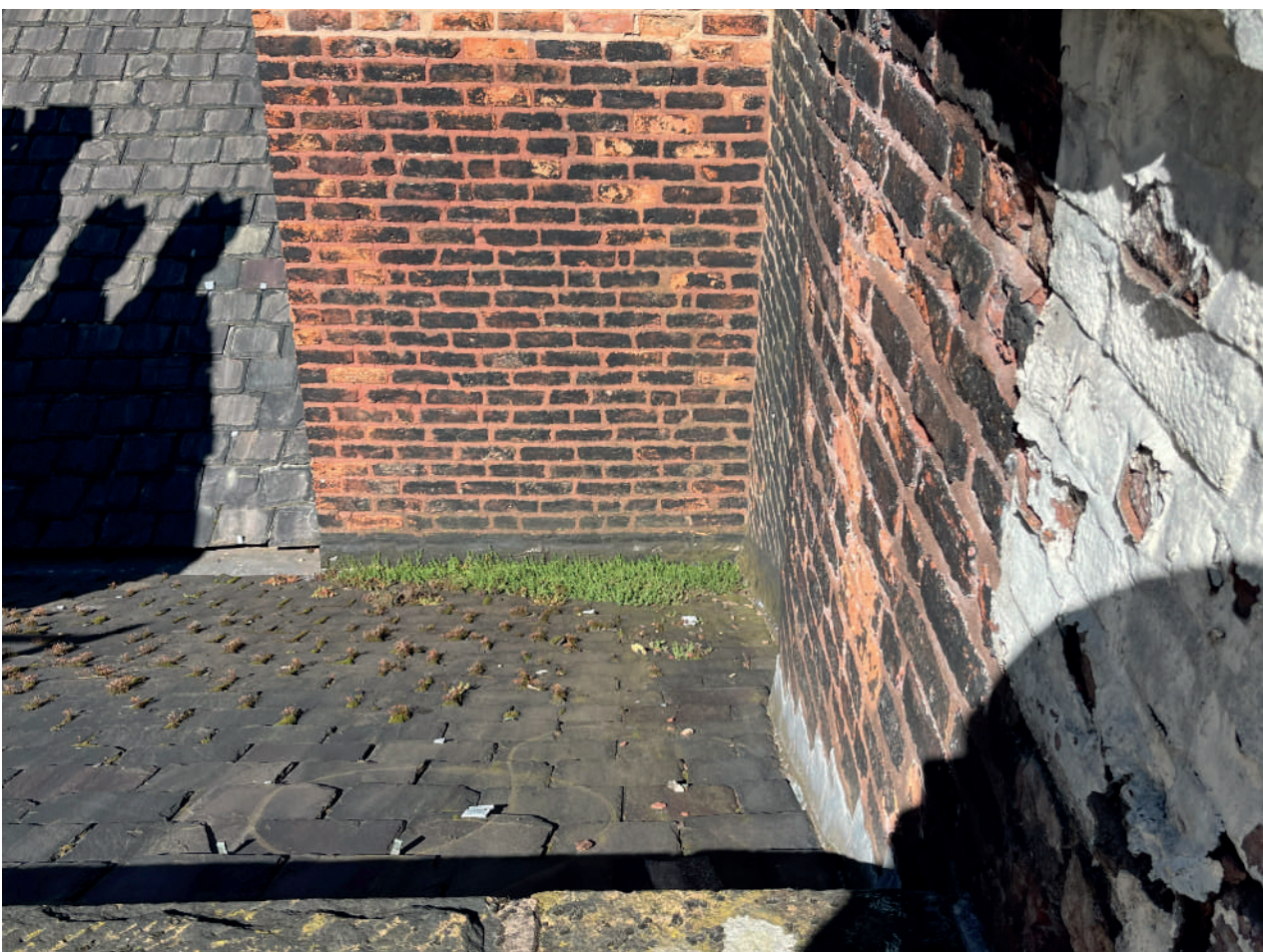
Flashing renewal required
