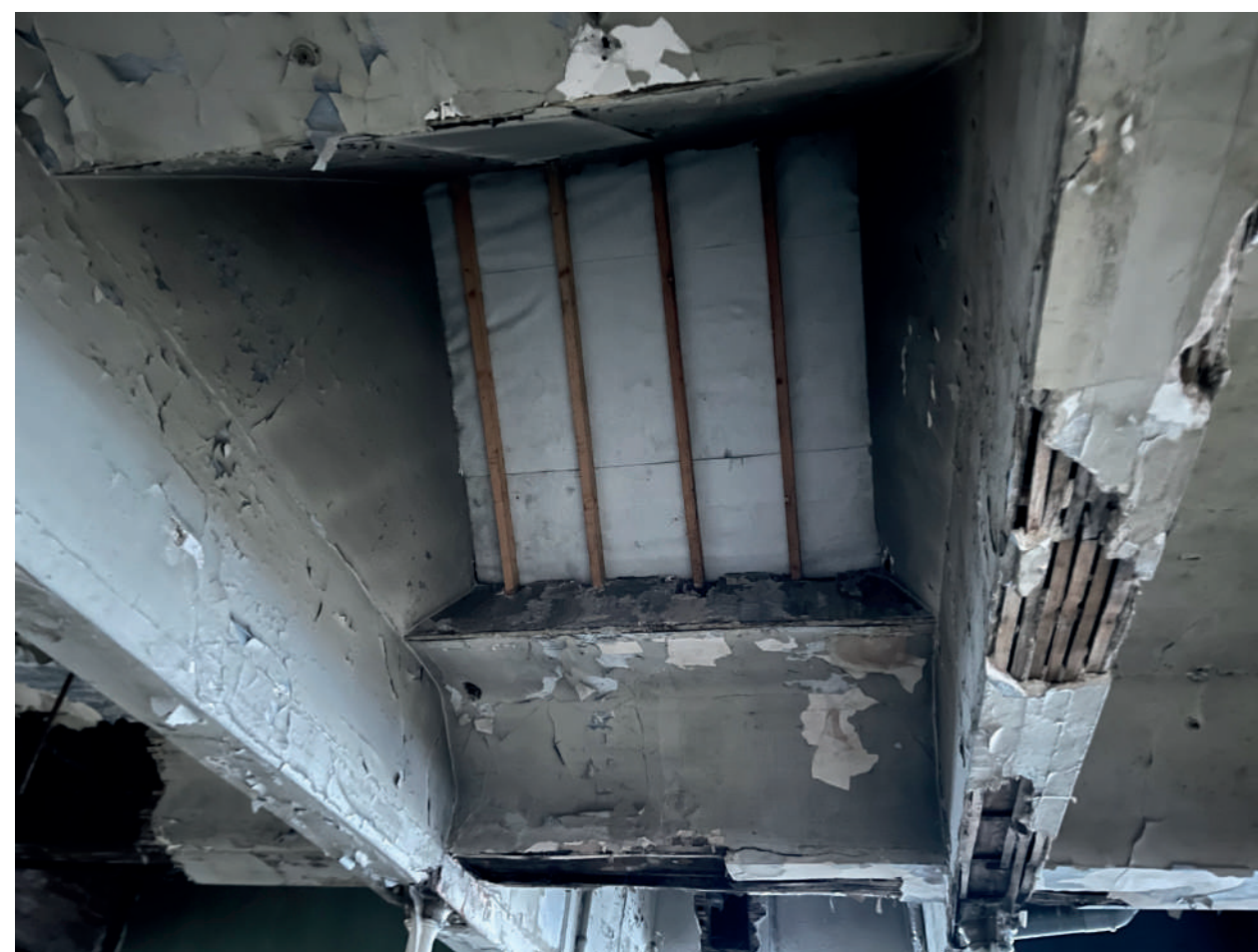
Previous roof repairs seen internally. Sloped ceilings locally.
