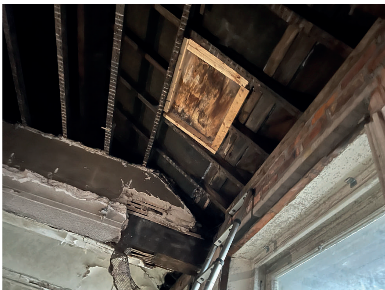
Rafters cut by previous owners to obtain access onto roof. These rafters will be repaired.
