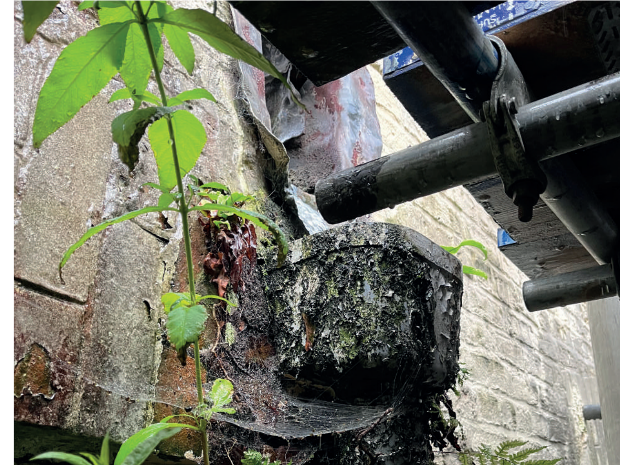
Gutter outlet lead renewal required, and replacement of plastic RWP and hopper with cast iron.
