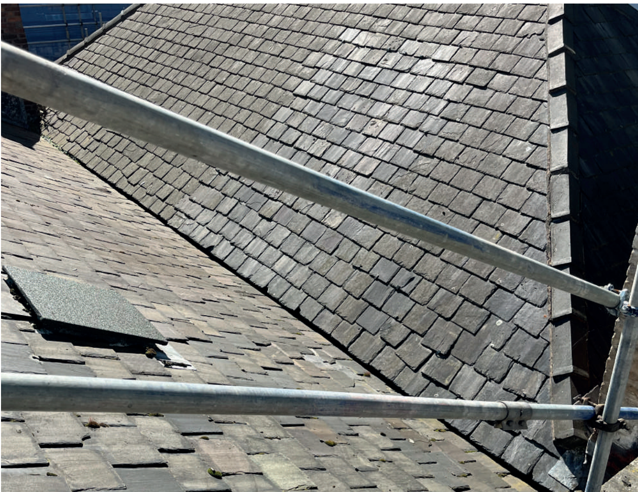
Slates installed incorrectly, blocking valley gutter below.
