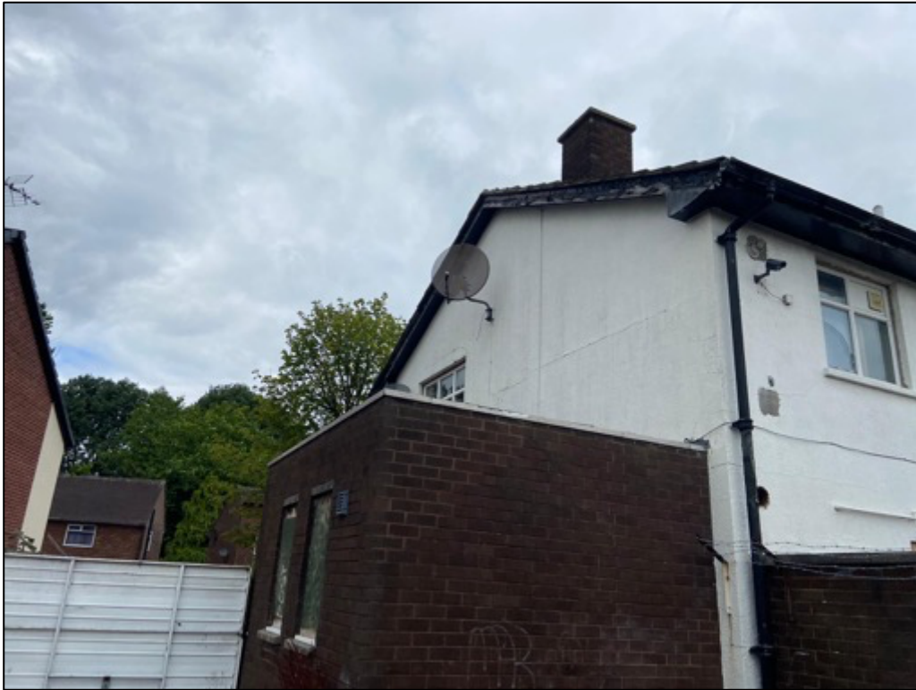
Photograph 3; The wooden fascia lining features some cosmetic damage due to age, but this does not affect the structural integrity of the roof and no openings were noted. Attached single-storey sections were more recently added and offer no ecological importance.
