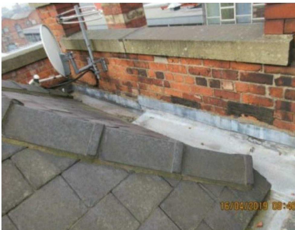
Figure 16: Looking west at the current aerial/satellite dish, located to the mid-south of the parapet. (Source: ProAV)
