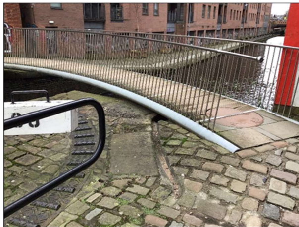
Q 11 - Gap between the lock access area railing and the footbridge railings.
