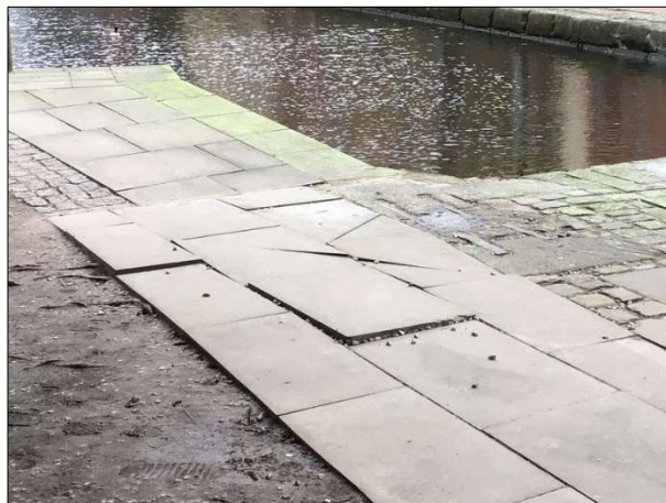
Q27 - Uneven paving near the reach pole station.
