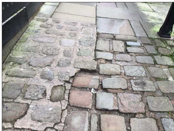
Q27 - Uneven section of cobbled paving near the footbridge over the canal.
