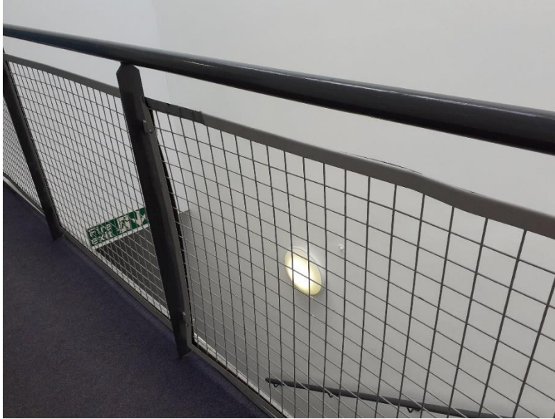
Damaged panels to balustrade.
