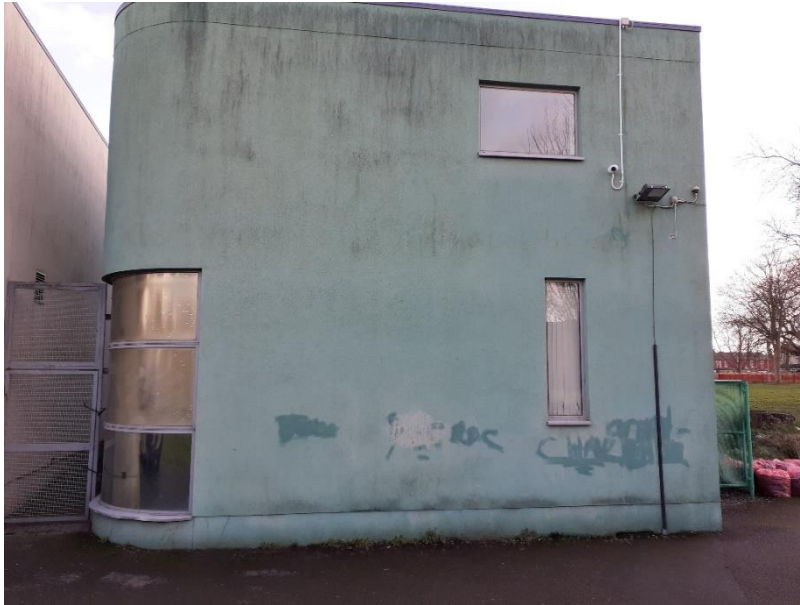
Stained cladding, vandal damage at low level
