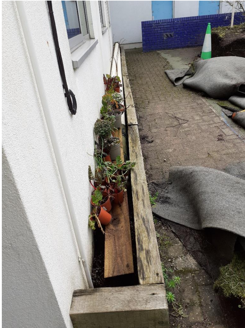
Soil in planter above DPC level
