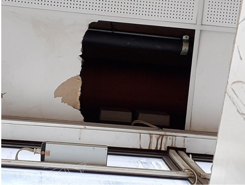
Water damage at high level.
