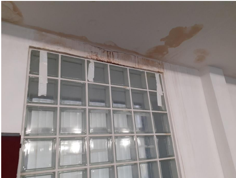
Rusting of lintel over opening.
