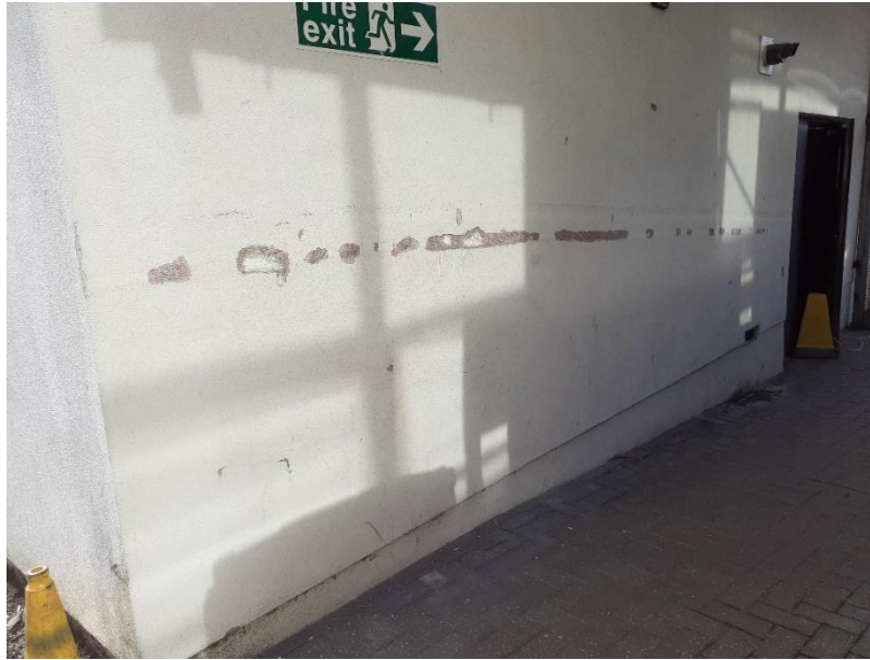
Typical damage to cladding panel
