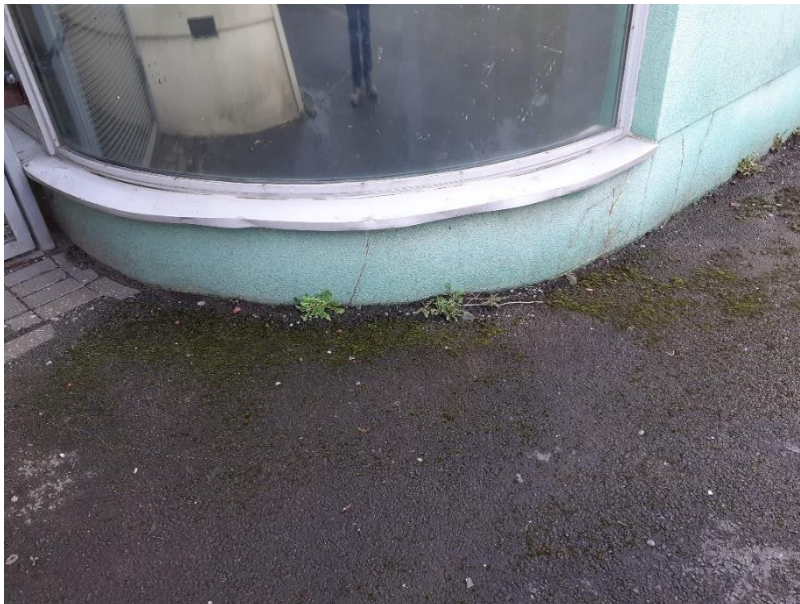
Vandal damage to sill
