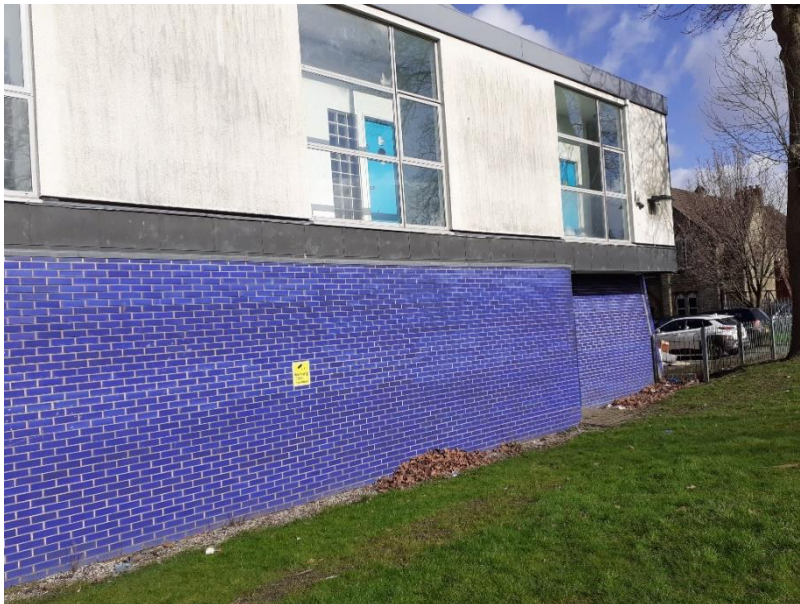
Stained cladding panels
