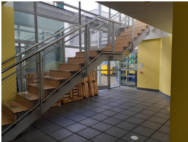
Headroom compromised below stair.
