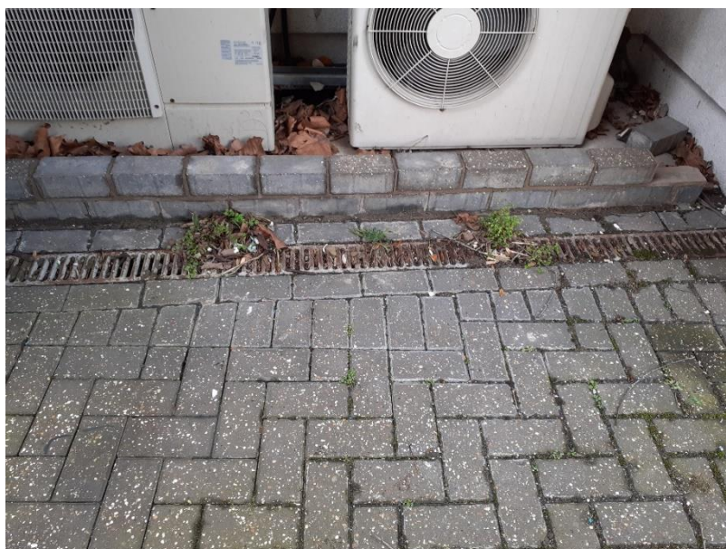
Blocked channel drain
