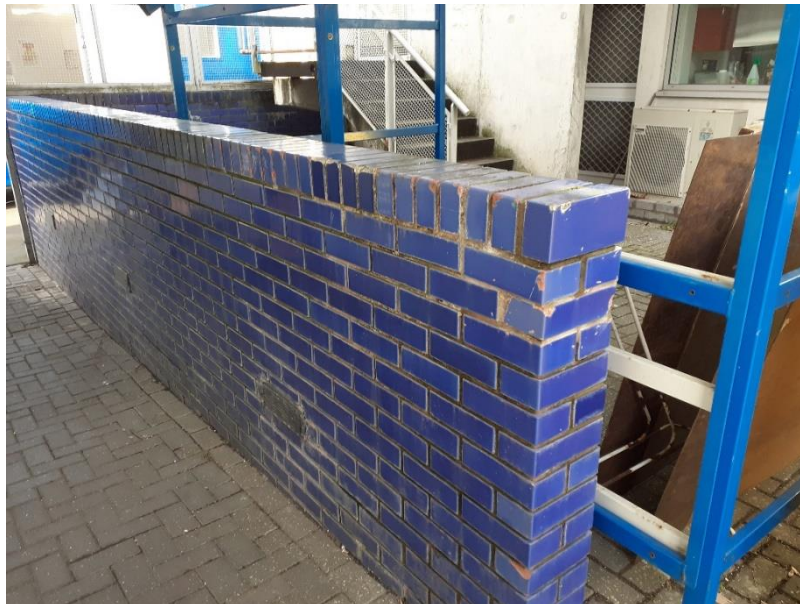
Damaged glazed bricks
