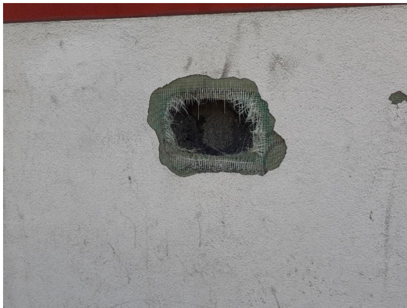
Typical hole in cladding
