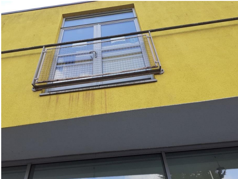
Corrosion of Juliet balcony
