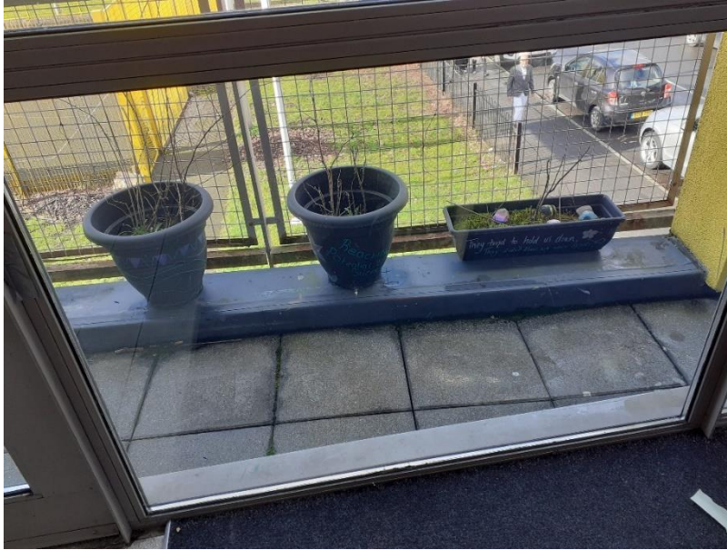
Decaying seals on curtain wall.
